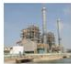
Combined Cycle Natural Gas
