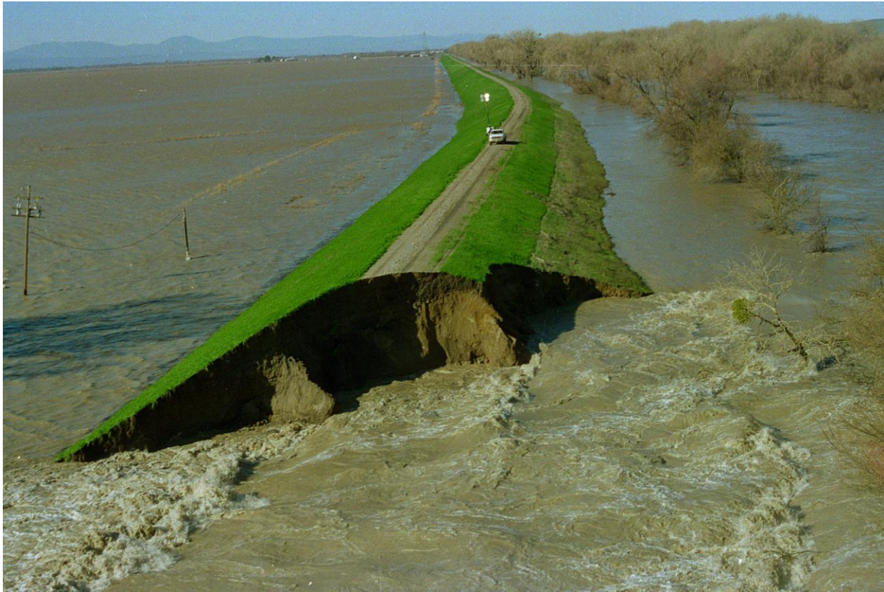
California Department of Water Resources Flooding - Levee damage
