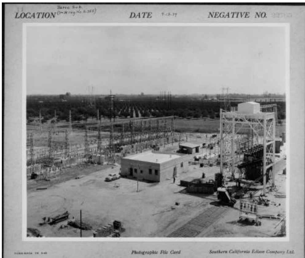
Barre Substation, under construction, September 13, 1939; Copyright: Southern California Edison Photographs and Negatives collection of The Huntington Library (Call No. 2-22765 / Image No. SCE_2_22765).
