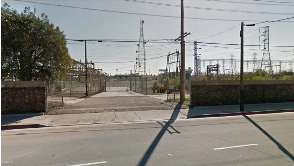
View south to main entry area and control house from West Cerritos Avenue
