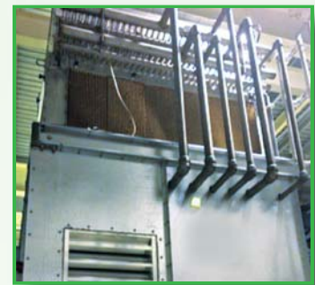
Evapcold units in the Wilson E. Bradley R&D Center, Taneytown, MD
