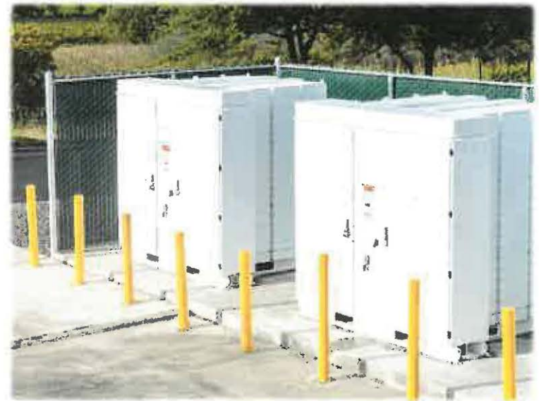
0.5 MW Tesla Battery Storage Installation
