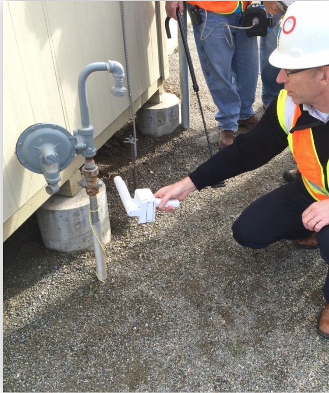
Using the handheld methane detector to pinpoint simulated leaks at Livermore training center (December 2014)
