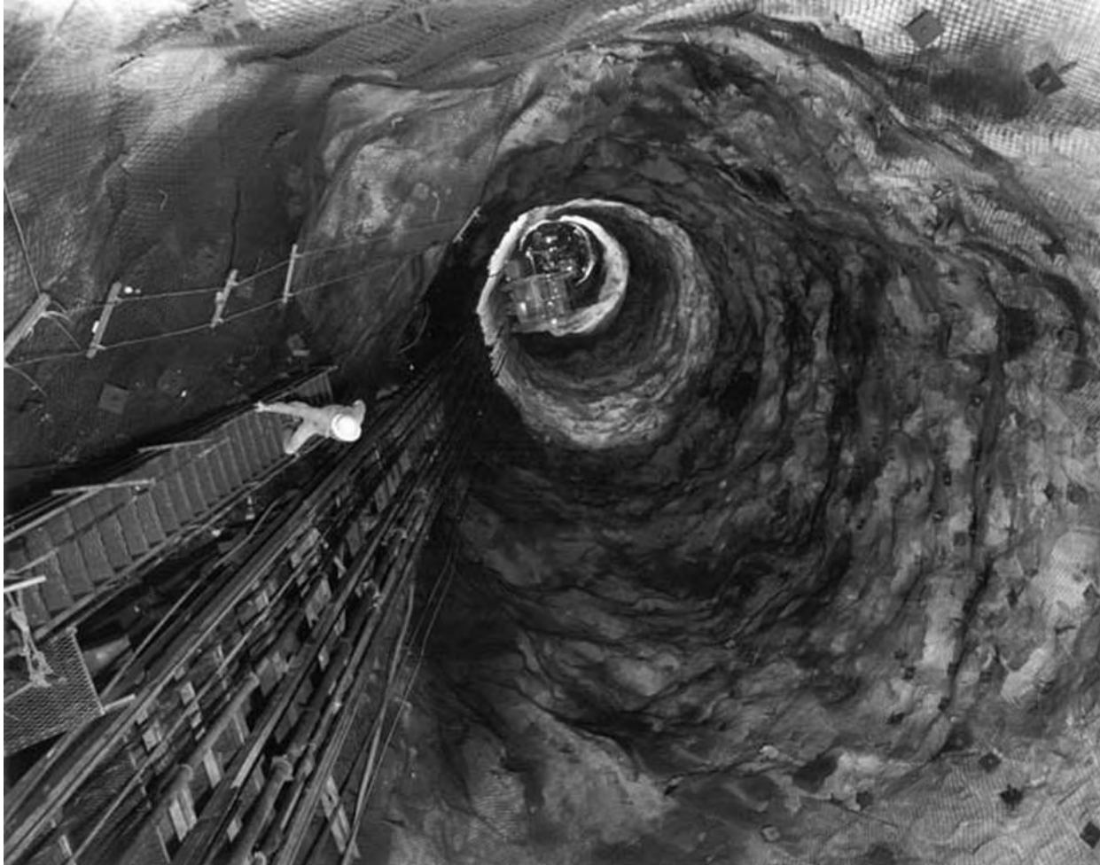
Inside the 27 foot diameter penstock that drops water 1,665 feet between Sierra Nevada lakes. Helms Pumped Storage Project cost $400 million and provides peak power then pumps water back uphill in the slack time. It is the partner facility to Diablo Canyon Nuclear Power Plant. August 22, 1980 PG&E photo
