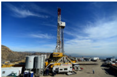
Crews at work last month on a relief well near Porter Ranch in California.
