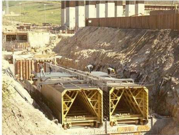
Robust Construction of DCPD twin cooling water tunnels noted by Bechtel during Nov. 18, 2014 meeting
