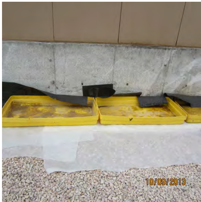
U1 Lube Oil/Eliminator
