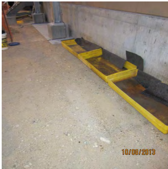
U3 Lube Oil/Mist Eliminator
