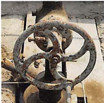
Undocumented Petroleum Feature in Survey Area
