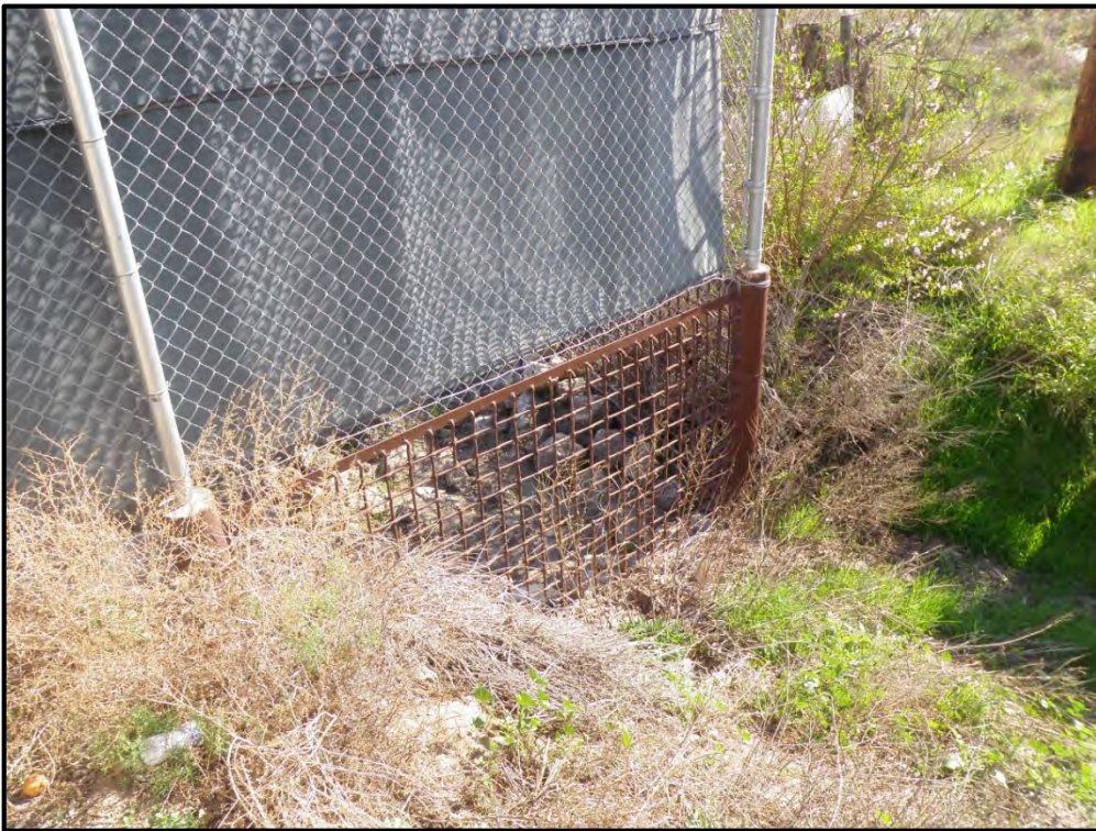
Figure 7. Northeast end of ditch at the in the southwest corner of the Granite facility; March 1, 2016.
