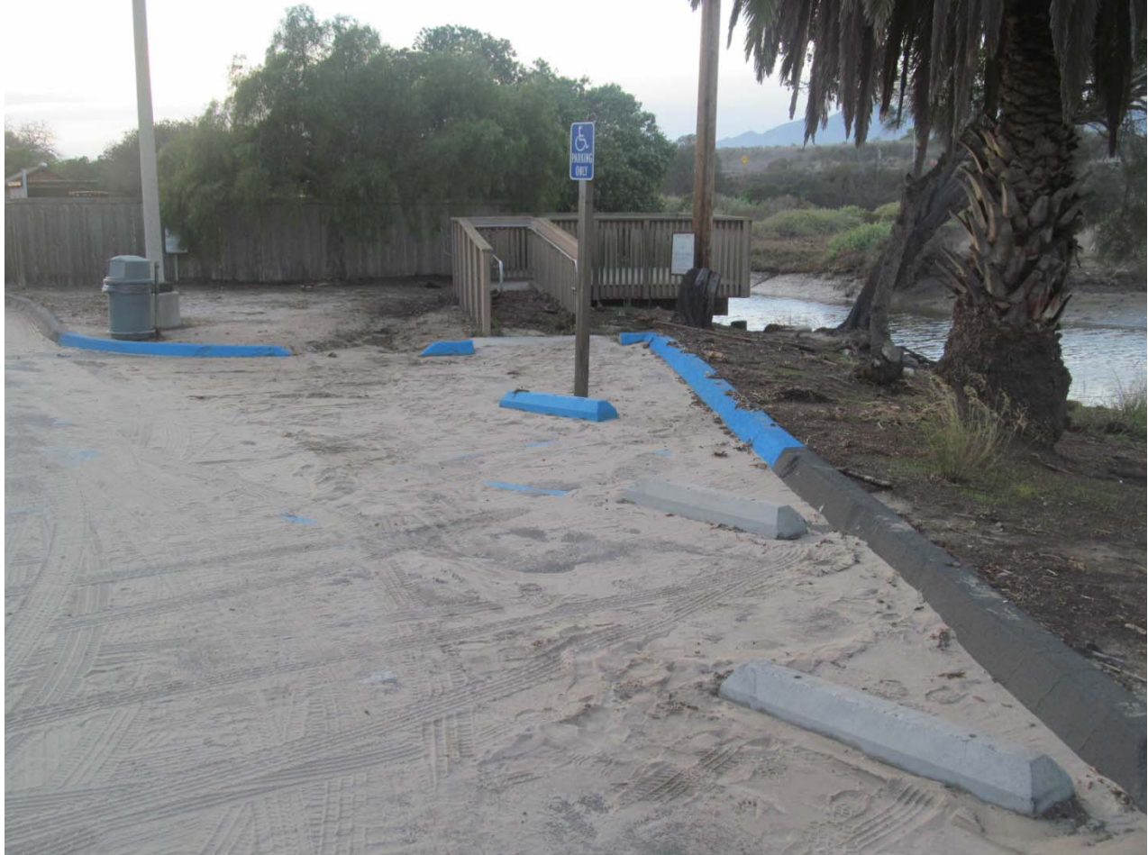
Figure 4E. Sand deposited from wave overtopping event on March 1 st at the back of the parking lot. Photo taken March 3, 2014 by David Revell.
