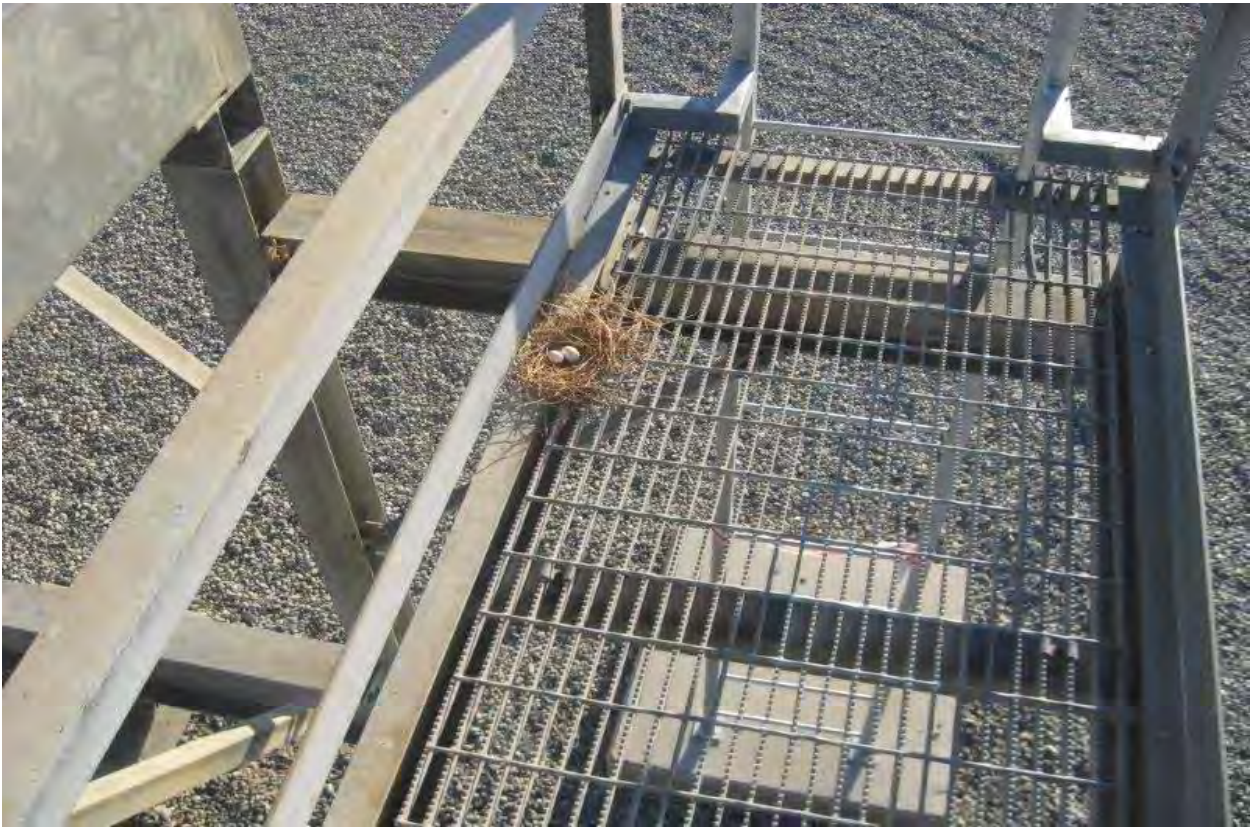
Photo 45, Eurasian dove nest on fin fan cooler, 9-25-15.
