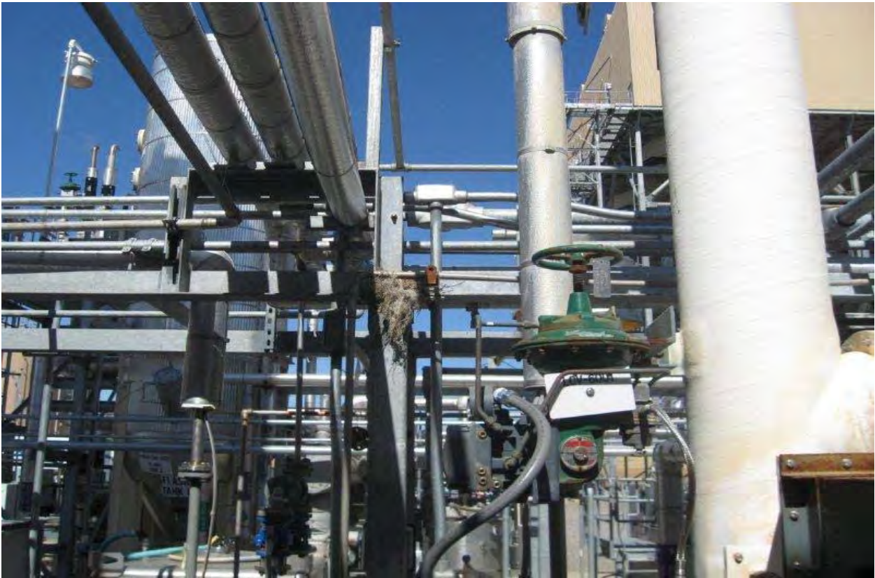
Photo 35, of typical nest situation in CGS piping, this was observed throughout the CGS site, 6-1-15.
