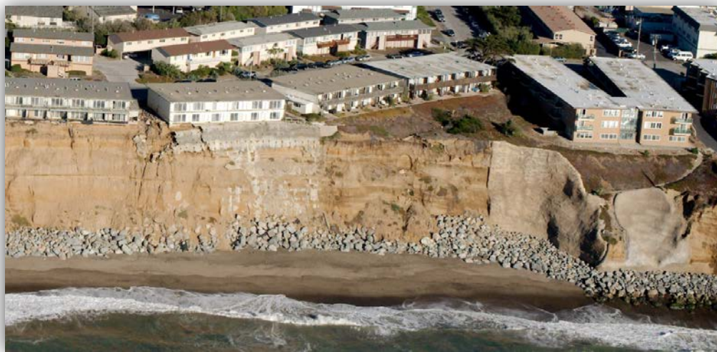
Figure 6. Photo of Esplanade Apartments threatened by cliff erosion in 2013 in Pacifica, CA. ( Source: California Coastal Records Project )
