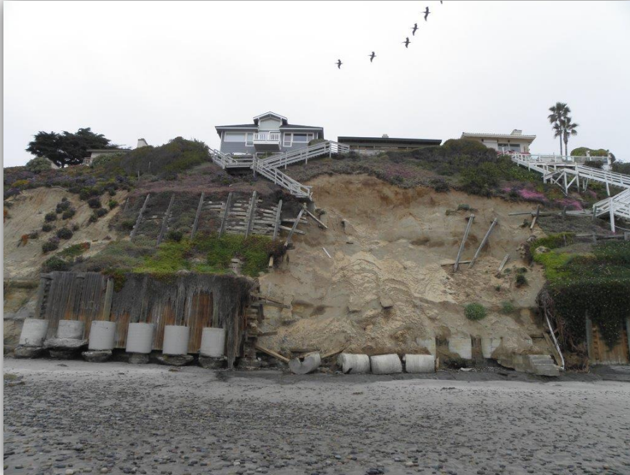
Figure 19. Photo depicting eroding bluff and exposed caissons in Encinitas, CA. (Photograph by Lesley Ewing)
