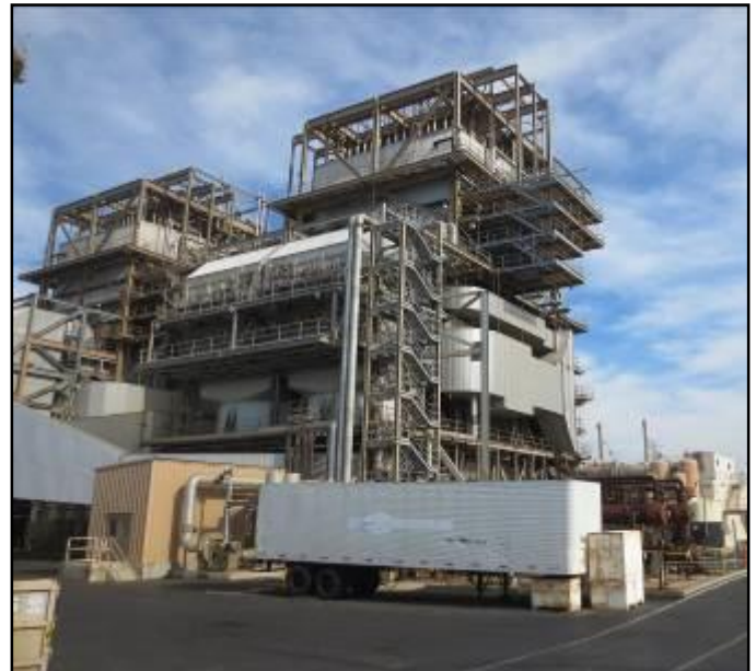
View of western and southern elevations facing northeast, displaying Units 1 and 2, and de-aerator system.
