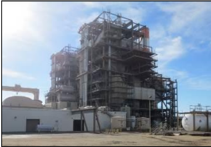
View of northern and eastern elevations facing southwest, displaying non-enclosed Units 1 and 2.
