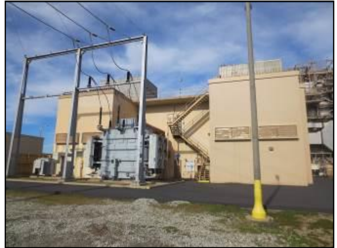
View of southern elevation of Unit 3 and connecting electrical lines, facing north.
