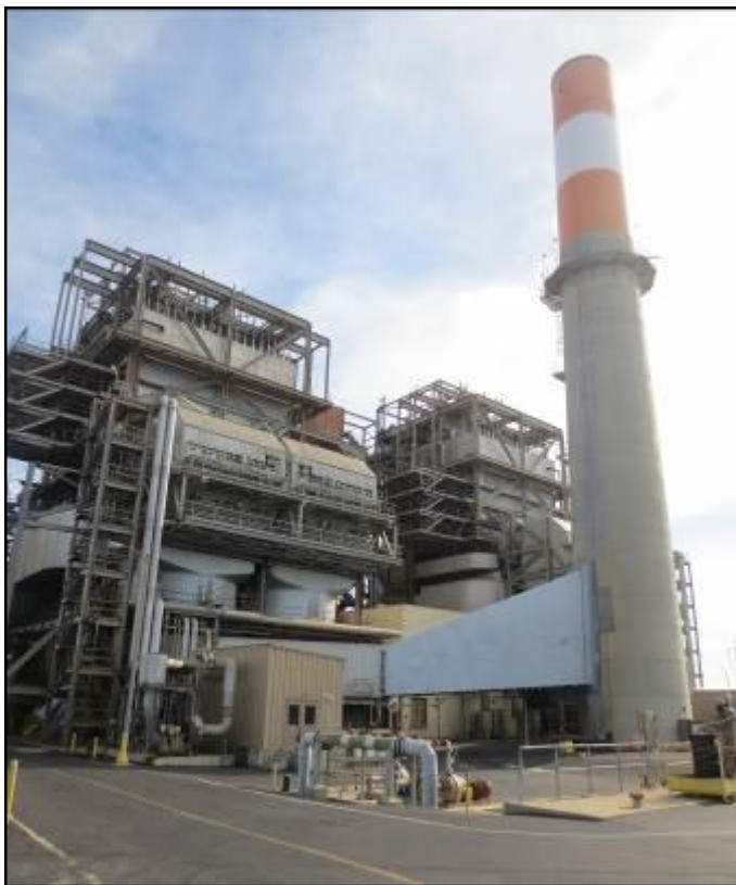
View of western elevation facing east, displaying Units 1 and 2 and steam plant stack.
