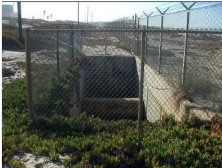
MGS Outfall mixing vault; view facing south.
