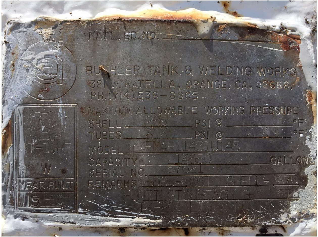
The original 1980 nameplate for the horizontal ammonia storage tank indicating that tank was designed for pressurized anhydrous ammonia, and its original nameplate pressure design was 265 psig.
