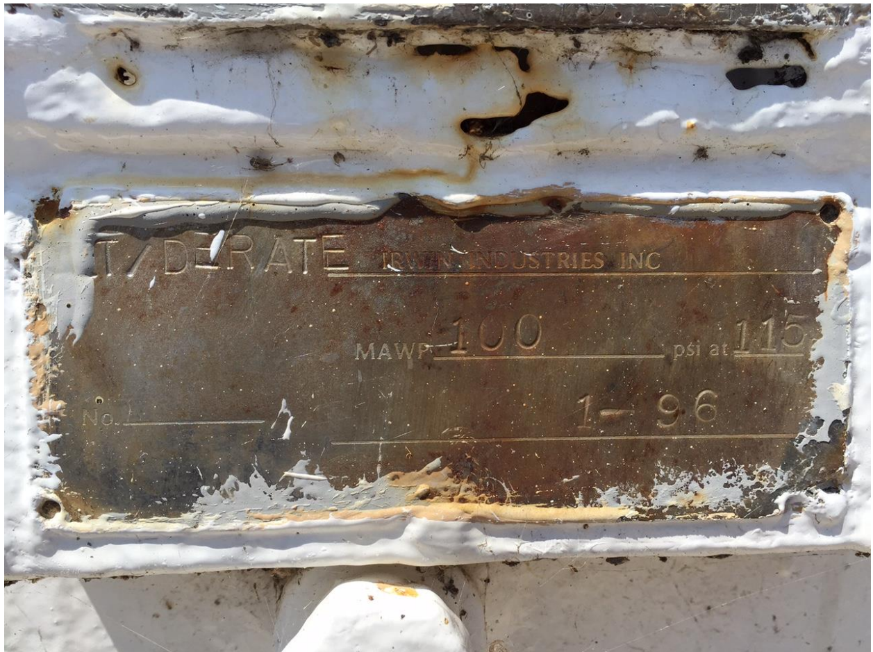
Nameplate on existing MGS ammonia storage tank showing current pressure rating of 100 psig @ 115°F on 1/1996. Pressure was downrated to 100 psig in 1996 from original 256 psig in 1980.
