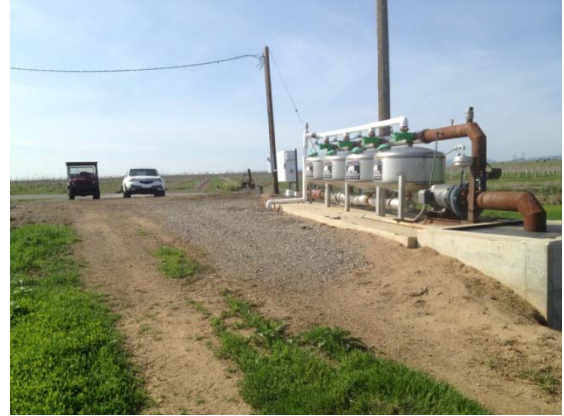
Photo 26, looking south at proposed water intake adjacent to existing structure. New intake line will be installed in cement box on right side of photo.
