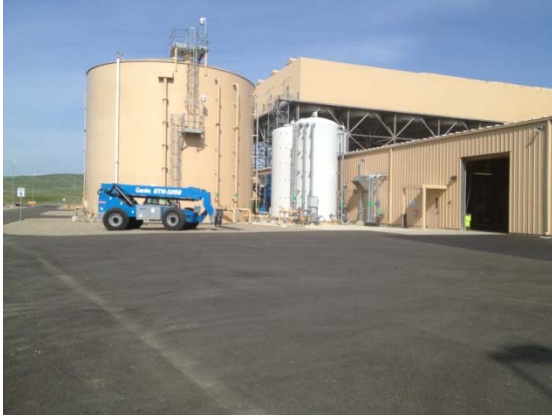
Photo 1, looking east within CGS. Waterline to enter into building in front of Gradall.
