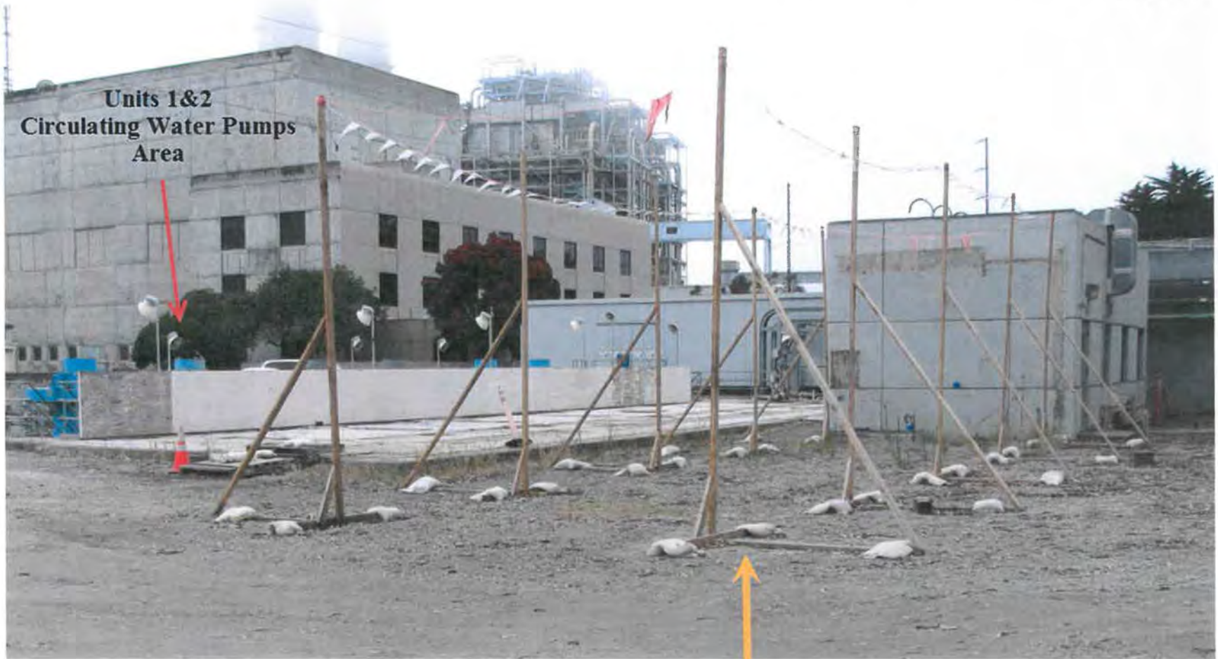
Figure 2 Concrete Slab & Building Location for VSDs Variable Speed Drive Controls Project Dynegy Moss Landing, LLC
