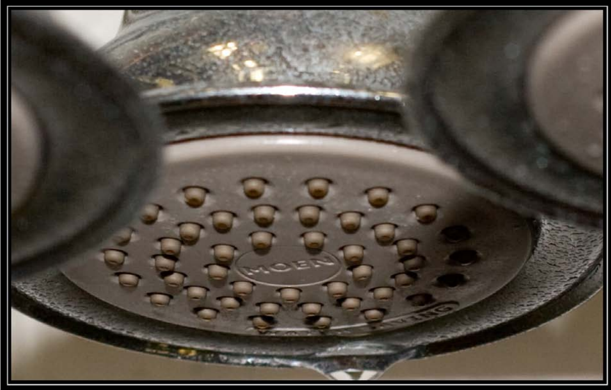
Figure 6-4C. Showerhead 4 on seventh day of testing with soft well water (<1 grain per gallon)
