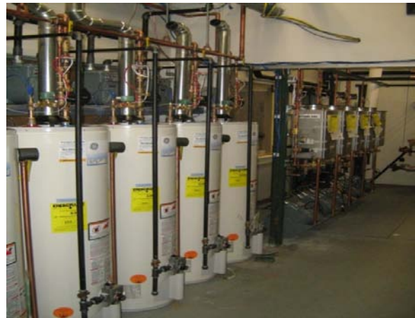
Figure 4-4. Gas Water Heaters
