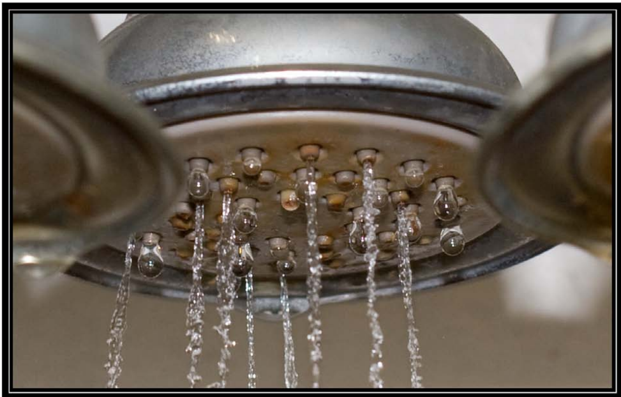
Figure 6-9D. Showerhead 9 on seventh day of testing with hard well water (28 grains per gallon) showing spray pattern. Battelle testing for Water Quality Association. May 1, 2009
