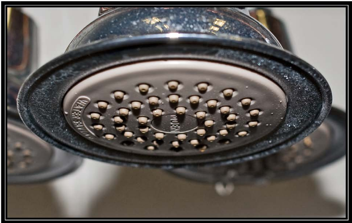
Figure 6-2A. Showerhead 2 on fourth day of testing with softened well water (<1 grains per gallon) showing condition of nozzles. Battelle testing for Water Quality Association. April 28, 2009
