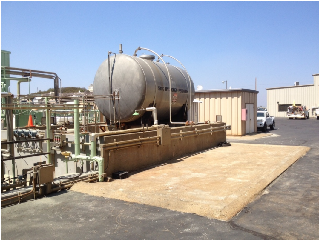
Attachment A Photos of Existing Hydrogen Peroxide Storage Tank and Containment Plant 1
