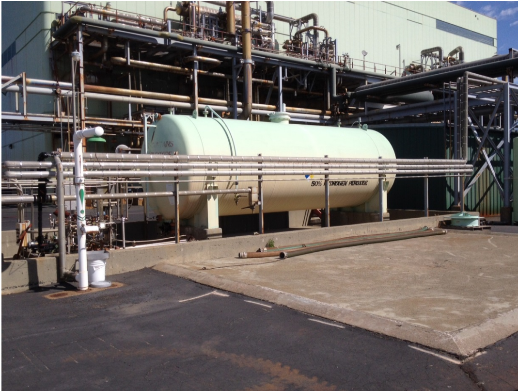
Attachment C - Photos of Existing Hydrogen Peroxide Tank General Location at Plant 2
