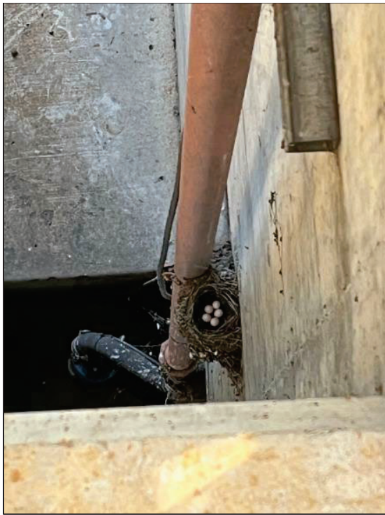
Photo 1: An active black phoebe nest with five eggs was found beneath the main steam pipe connected to the air-cooled condenser (ACC) on April 1, 2025.
