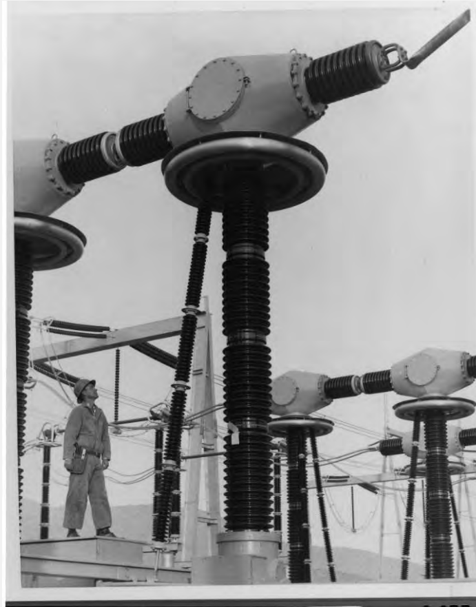
Exhibit 6. A substation maintenance employee stands beside one of the new 500kV air circuit breakers at the Vincent Substation (circa 1970).
