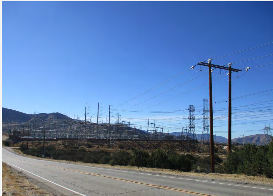
Photograph 2. SCE Vincent Substation, view to the southwest
