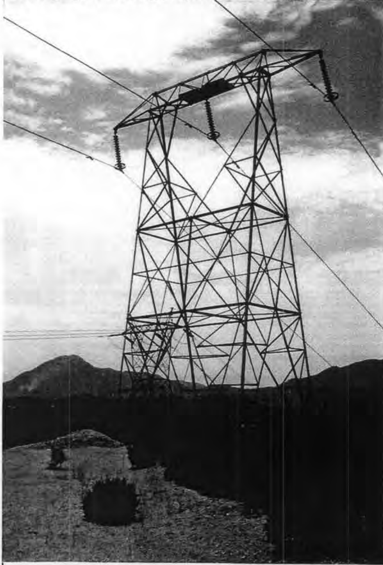
Description of Photo: Typical steel lattice transmission line tower
