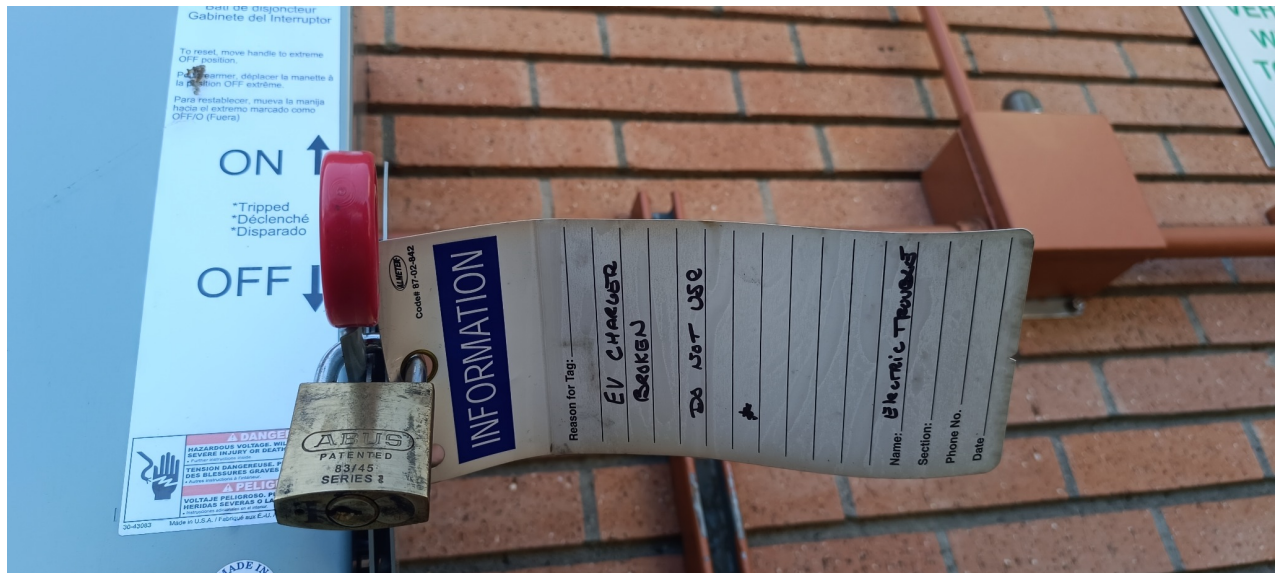
Exhibit N - Additional electrical equipment padlocked/tagged with handwritten notice indicating the EV charger is broken and should not be used. Station ID is not established by this image.
