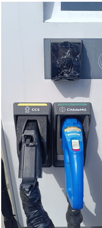
Exhibit G - Station 3741. Damaged charging hardware and visibly damaged interface/display.
