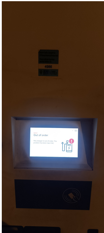
Exhibit B - Station 4986, September 10, 2026. Display states the charger is out of order.
