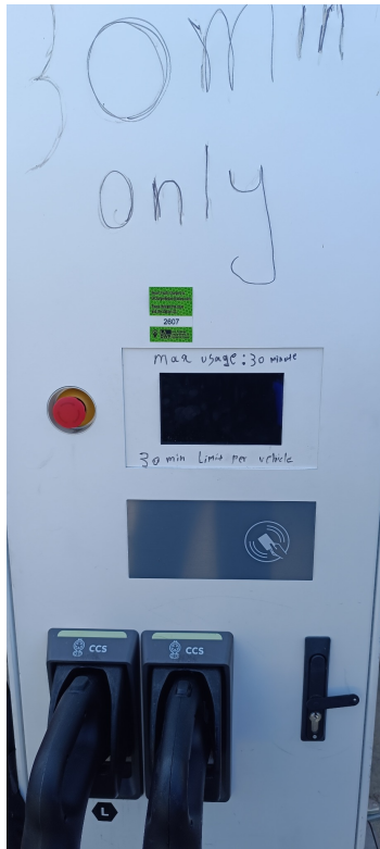
Exhibit M - Station 3676. Separate observation shows a CHAdeMO session delivering power, demonstrating reduced capacity rather than total station failure.
