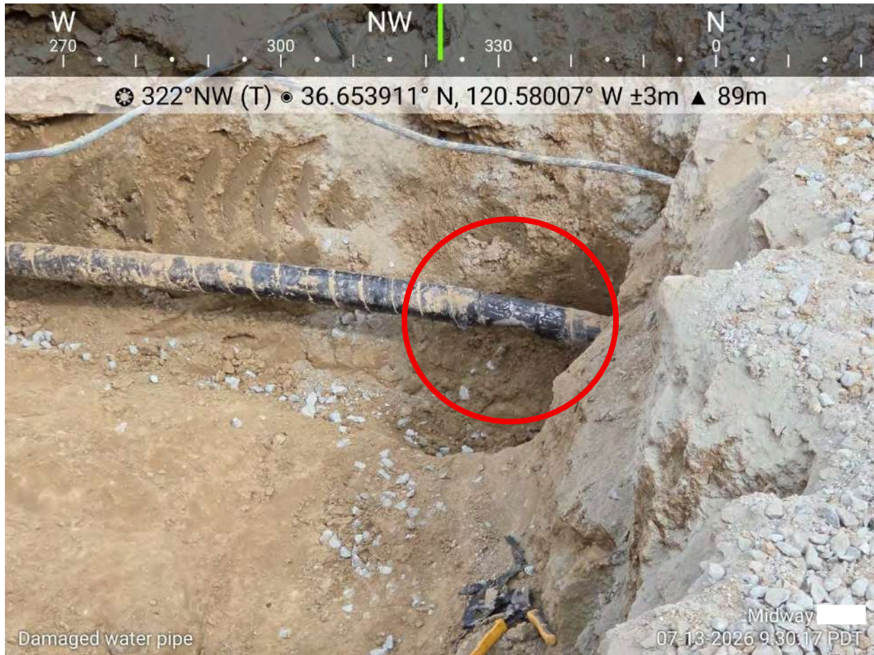
Damaged DI water pipe (red circle).
