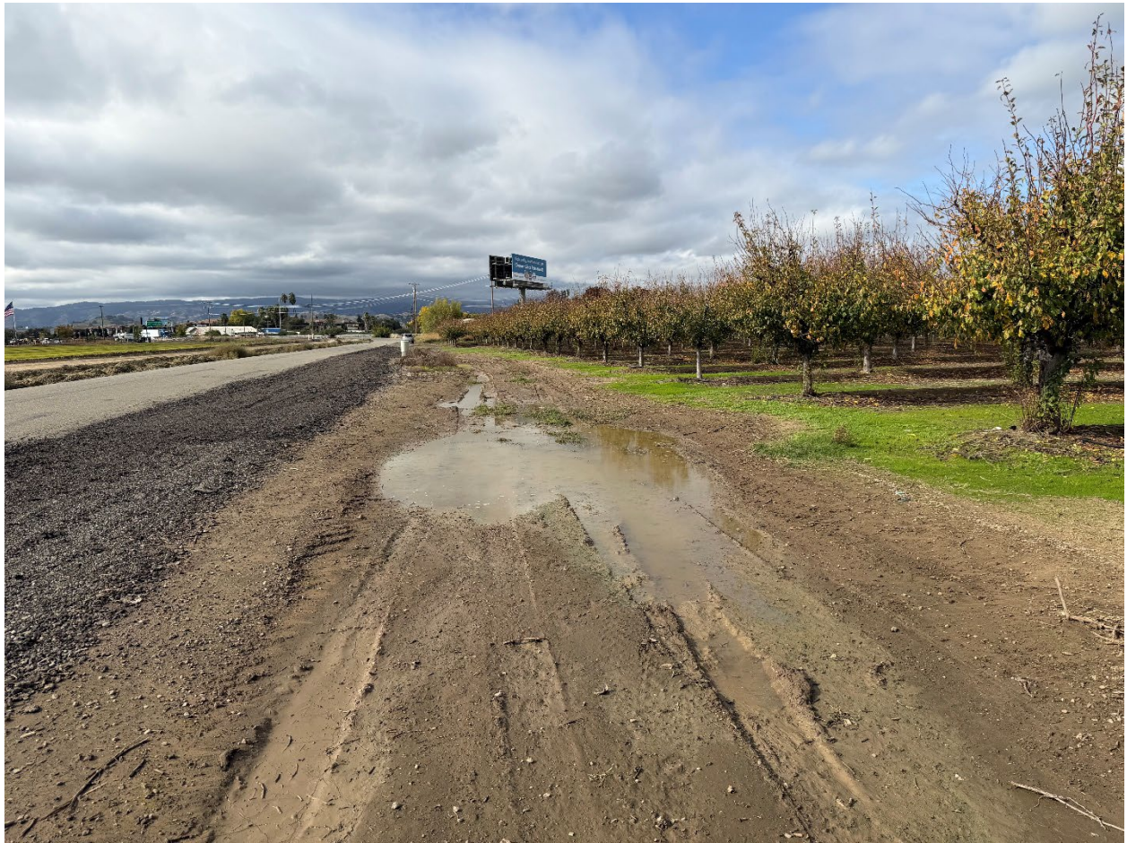
Photograph of HBC-2 road rut taken by Brent Helm on November 7, 2026 facing west.
