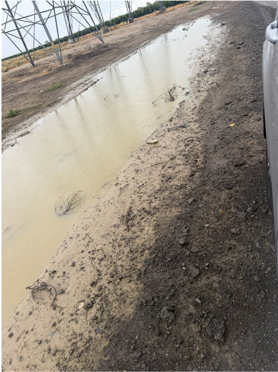
Photograph of HBC -1 road rut taken by Brent Helm on April 24, 2026 facing northeast.
