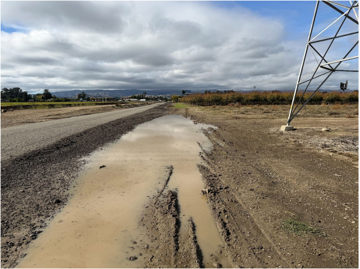
Photograph of HBC-1 road rut taken by Brent Helm on November 7, 2026 facing west.
