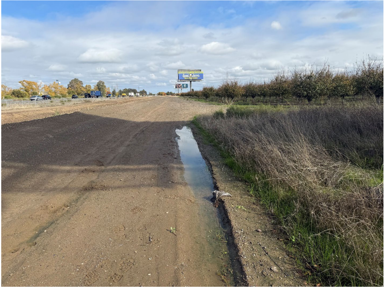
Photograph of HBC-5 road rut taken by Brent Helm on November 7, 2026 facing north.
