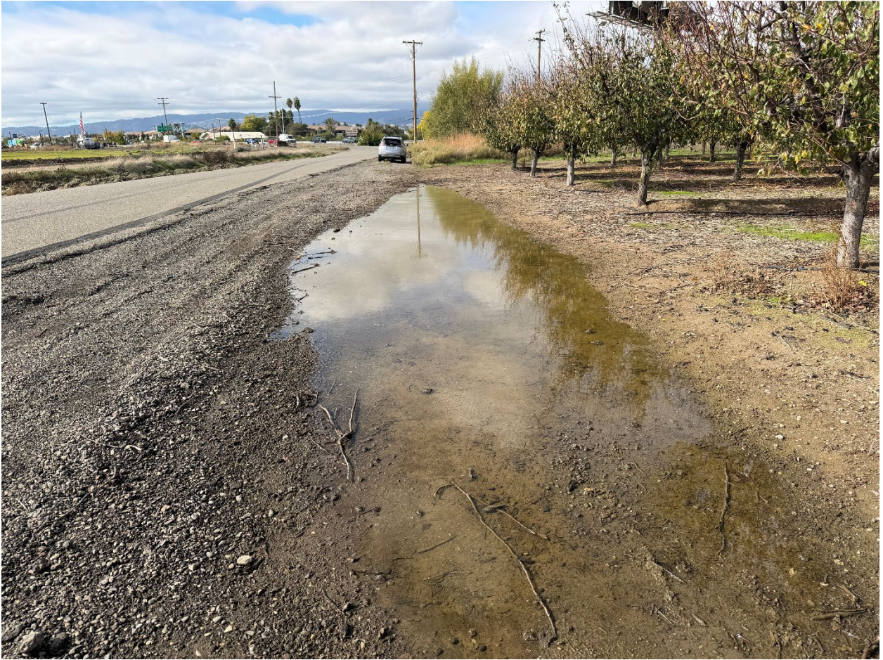
Photograph of HBC-3 road rut taken by Brent Helm on November 7, 2026 facing west.
