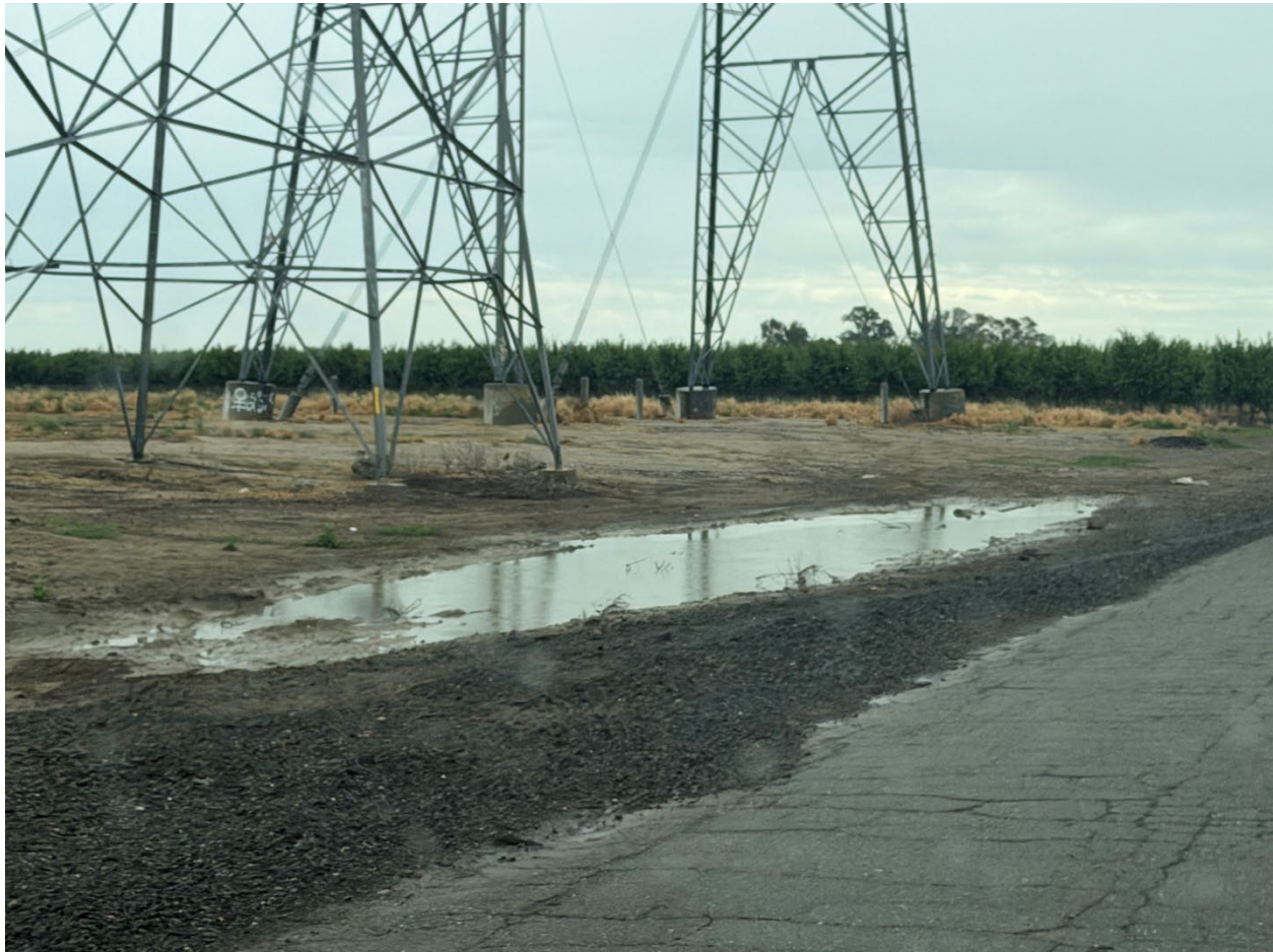
Photograph of HBC -1 road rut taken by Brent Helm on April 24, 2026 facing northeast.
