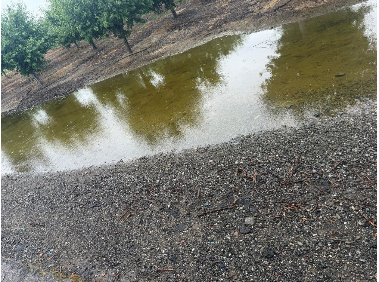
Photograph of HBC-3 road rut taken by Brent Helm on April 24, 2026 facing northwest.
