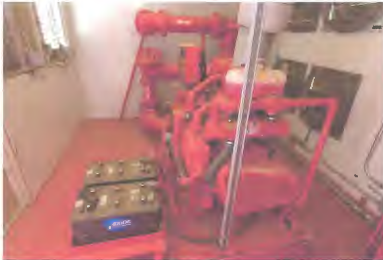
S-6 Emergency Fire Pump
