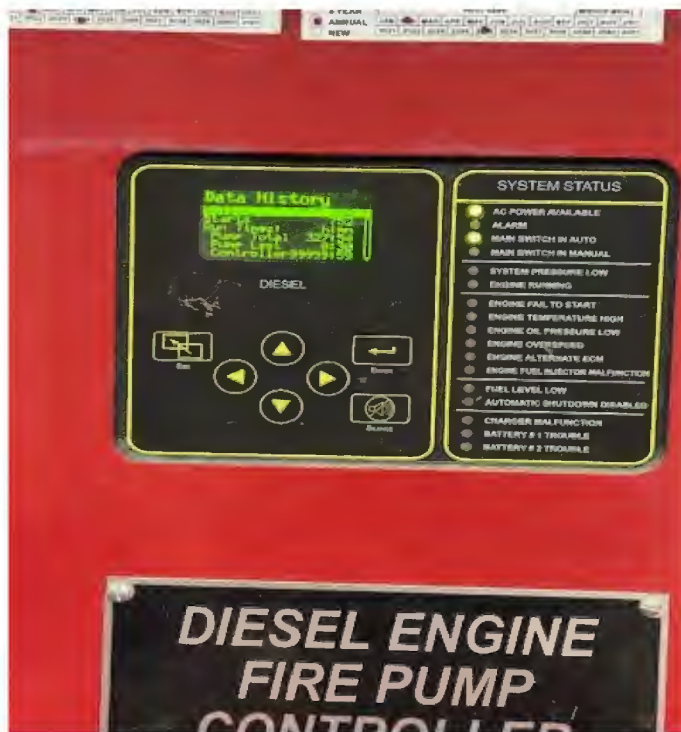
S-6 Controller, Showing Fire Pump Operating Hours
