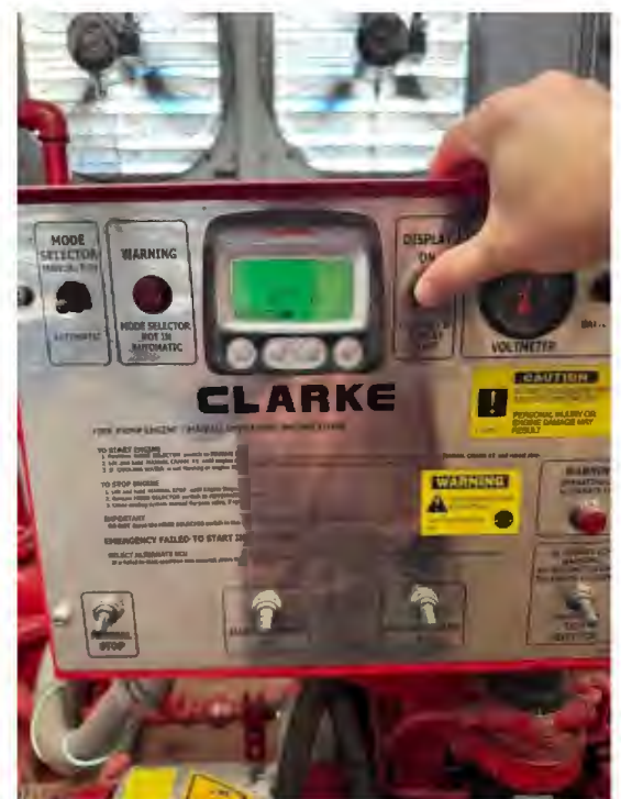
S-6 Fire Pump Engine Hours
