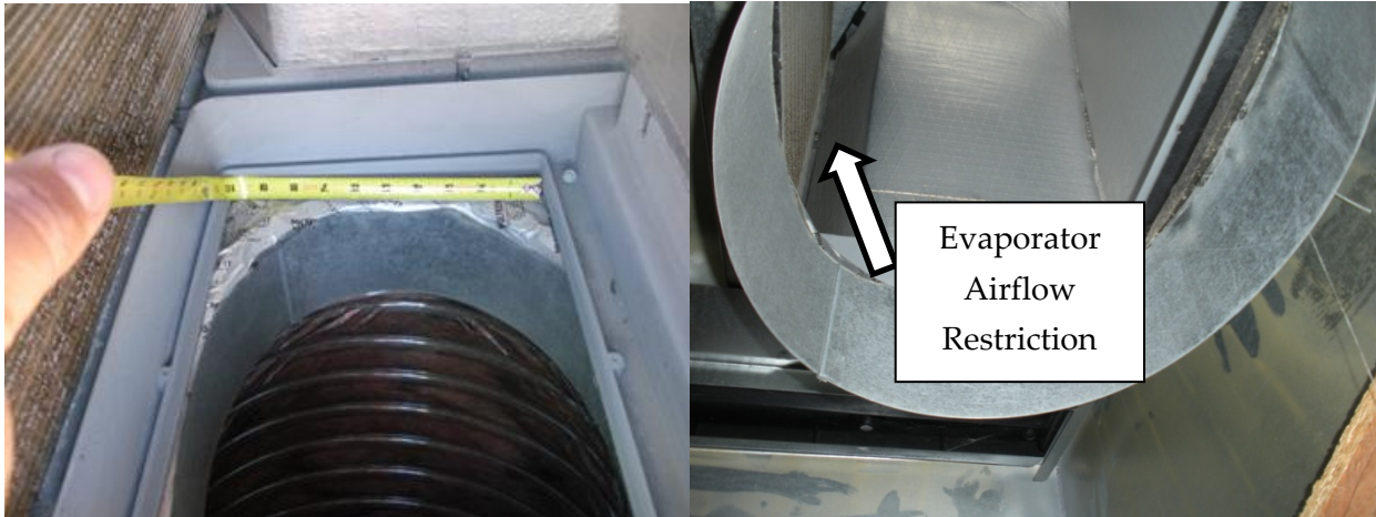
Figure 37: System 27—“Ovalized” Return Duct and Airflow Restriction to Evaporator Coil
