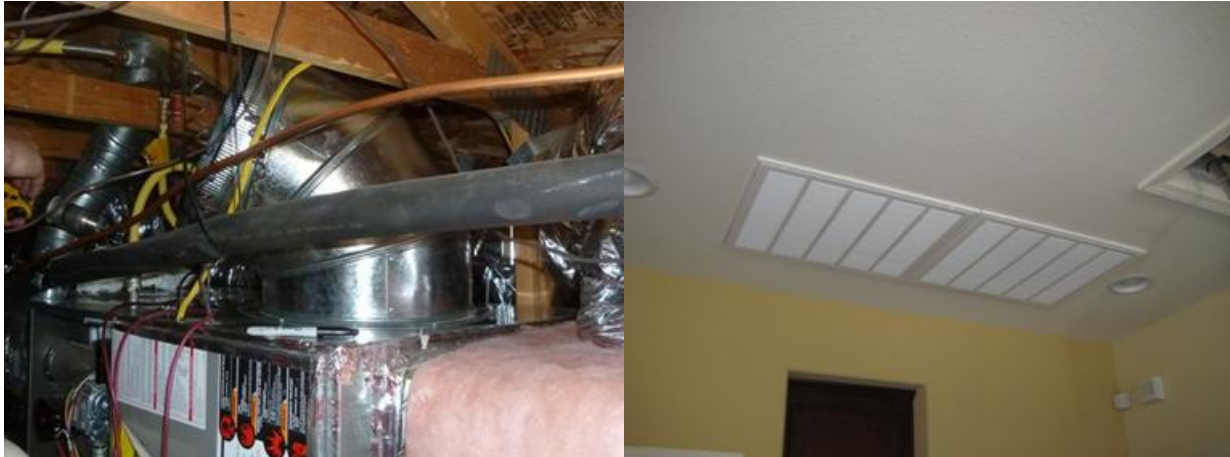
Figure 36: System 25—Metal Elbow Into Cabinet and New Filter Grille
