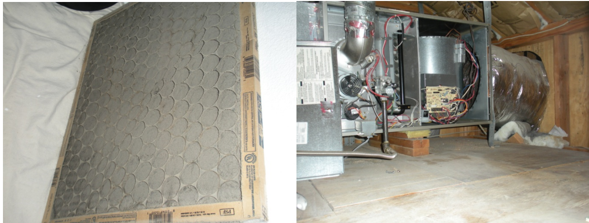
Figure 31: System 8—Clogged Filter and Original Return Duct Into “Bottom” of Furnace
