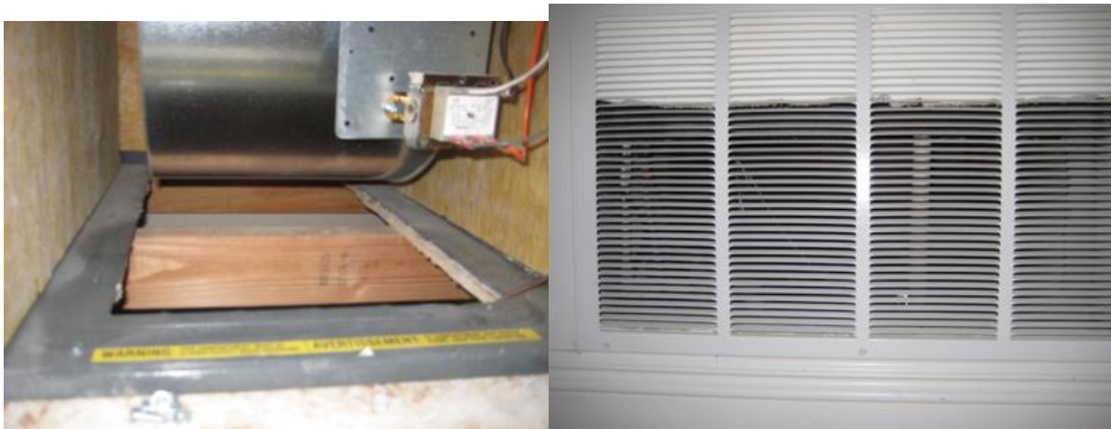
Figure 45: System 74—Poor Quality Installation: Restricted Return Grille Opening and Restricted Platform Opening
