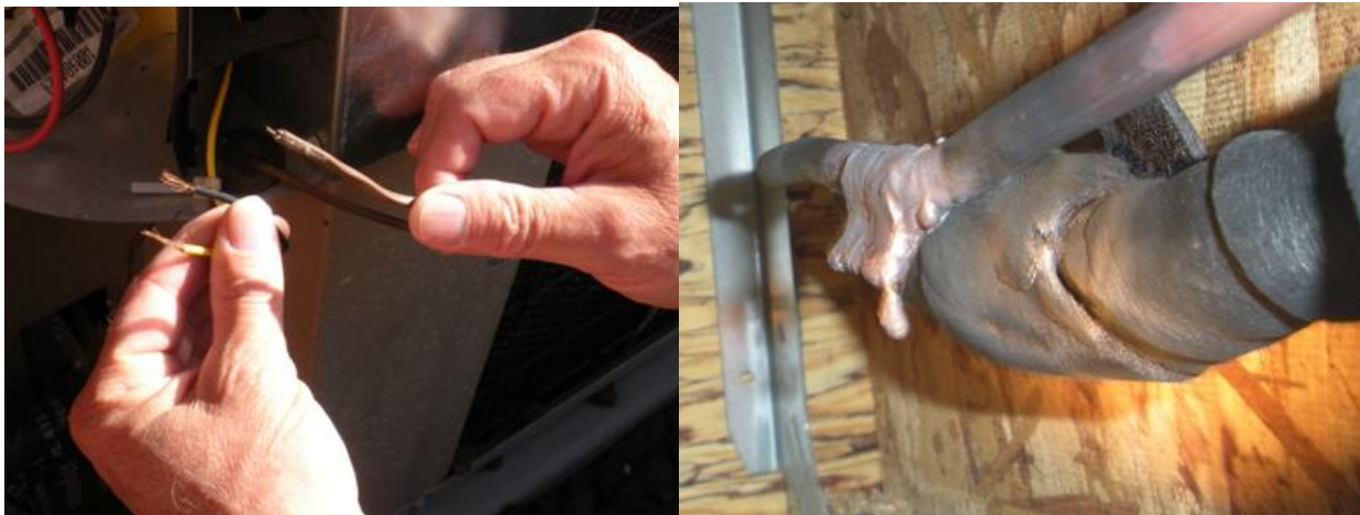
Figure 44: System 74—Poor Quality Installation: Control Wires Not Connected and Bad Brazing
