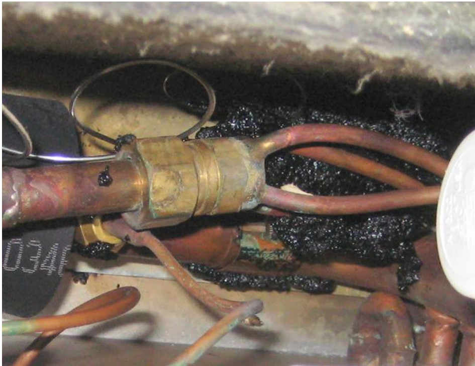
Figure 16: Unit 58—Melted TXV Bulb Insulation
