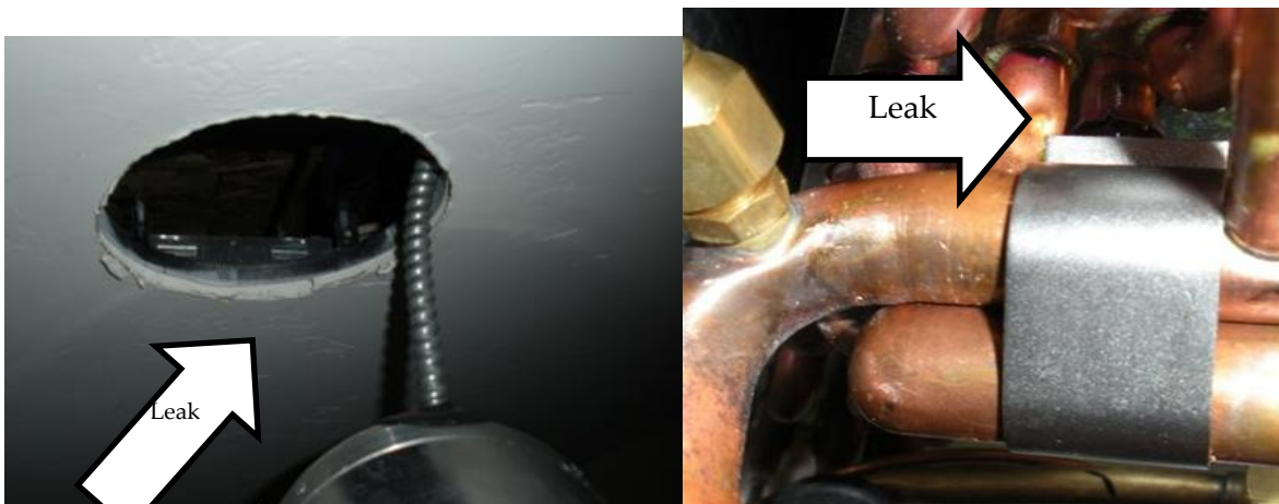
Figure 46: System 74—Refrigerant Leaks
