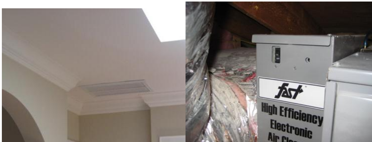
Figure 42: System 47—Original Return Grille Near Skylight and Side Feed “Bubble Wrapped” Return Plenum and Electronic Air Cleaner
