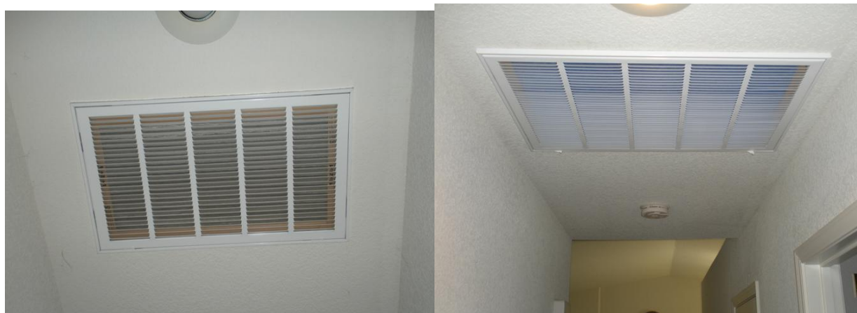
Figure 41: System 27—Original Return Grille With Pleated Filter and Enlarged Return Grille With “High Flow” Filter
