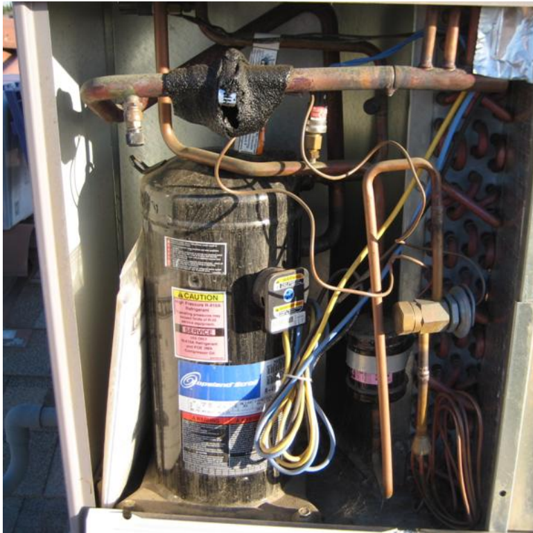
Figure 38: System 27—Compressor Compartment With Melted TXV Insulation
