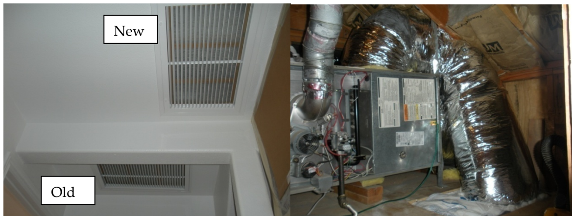
Figure 32: System 8—New Filter Grille Near Existing Grille and New 12 in. dia. Flex Duct Into Furnace Cabinet
