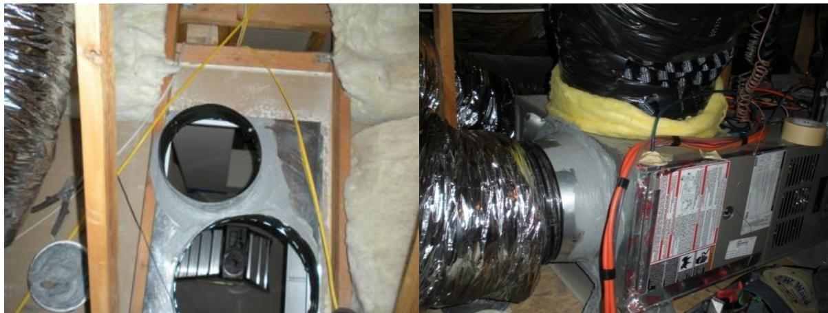
Figure 35: System 17—New Return Location and Double Ducts Into Blower Compartment
