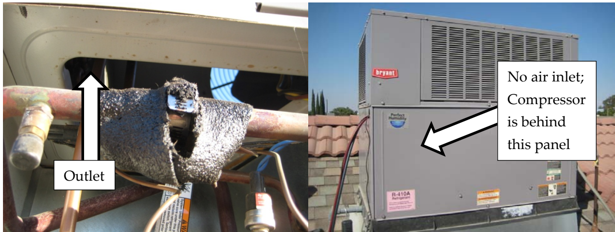
Figure 39: System 27—Compressor Heat Outlet With No Cooling Inlet
