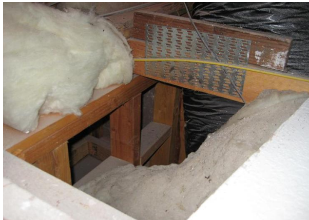
Figure 57: Leakage between Conditioned Space and Attic
