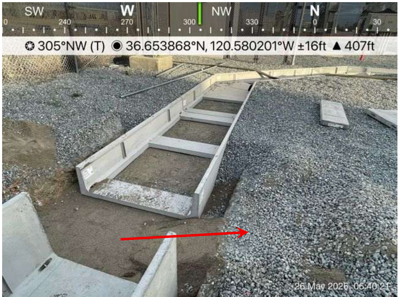
Earthen wildlife escape ramp in place.
