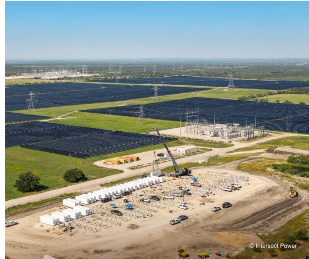
Darden Clean Energy Solar + Storage Project
