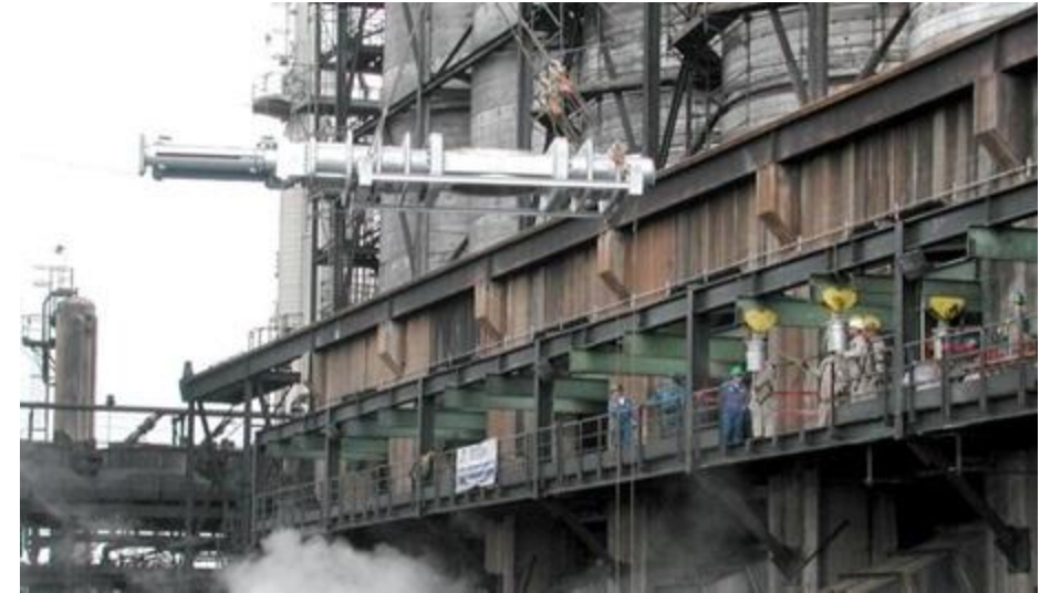
Source: Aegion Energy Services
