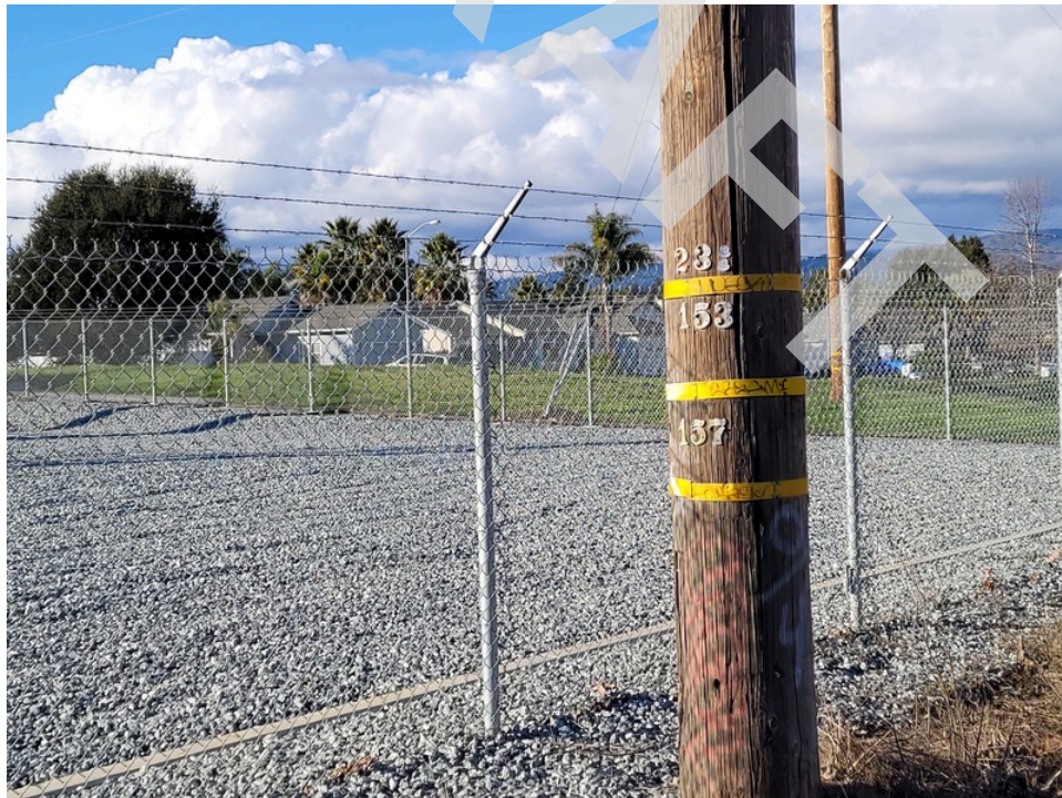
26. Utility pole northwest of the lease area
