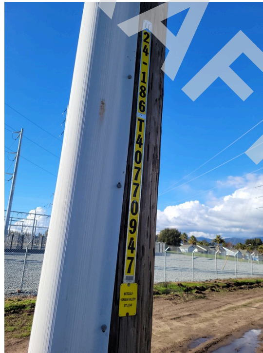
18. Utility pole at the northwestern end of the lease area
