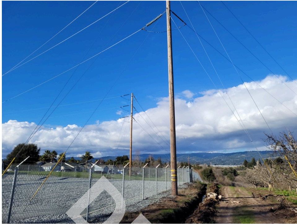
25. Utility pole northwest of the lease area
