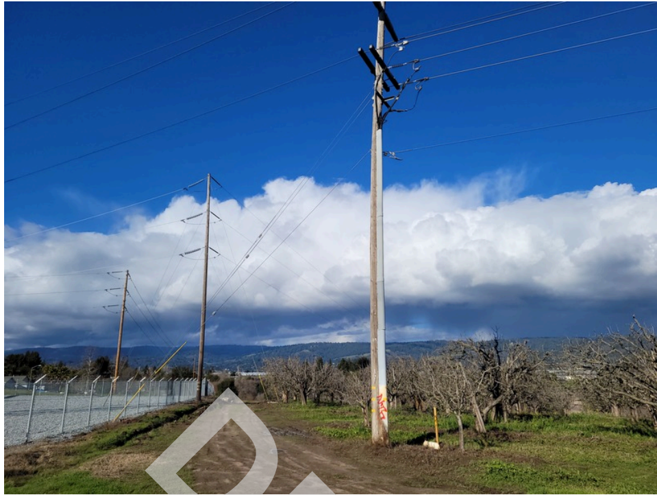
17. Utility pole at the northwestern end of the lease area
