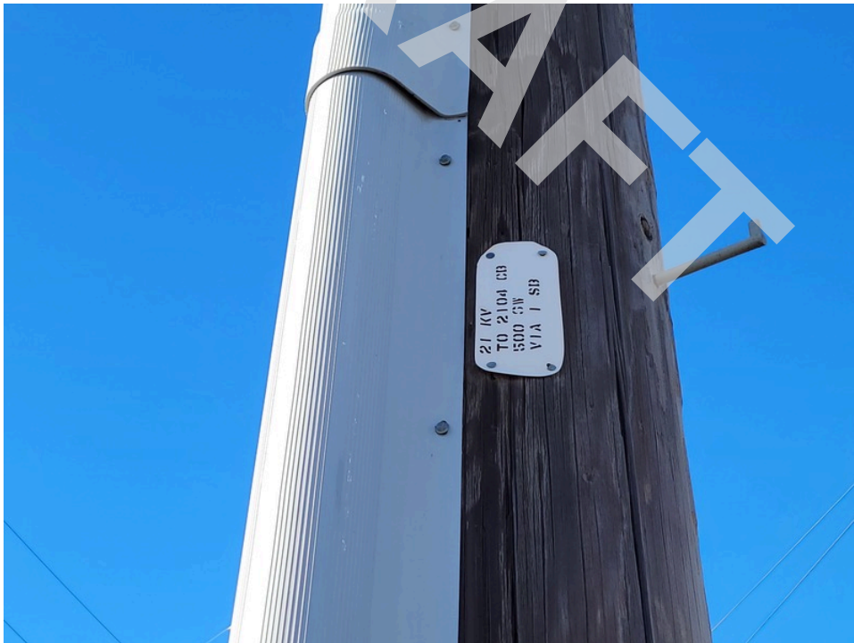
20. Utility pole at the northwestern end of the lease area
