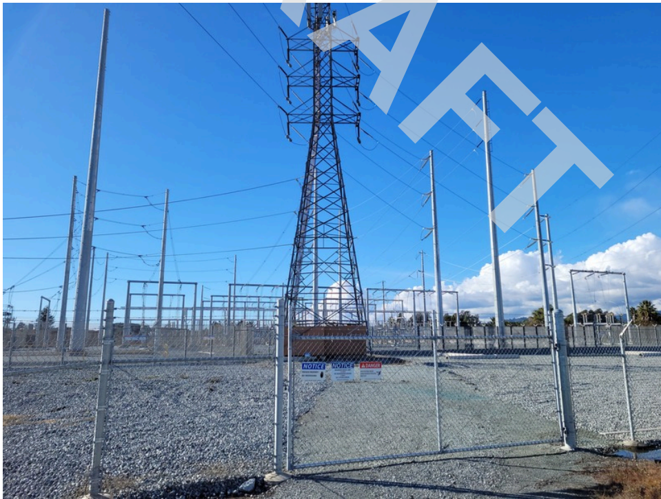
30. Green Valley Substation (76 Minto Road) adjacent to the northwest
