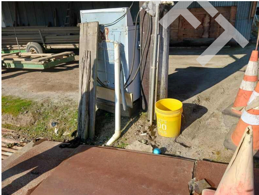
30. Washing machine attached to the "gray water" drainage system.
