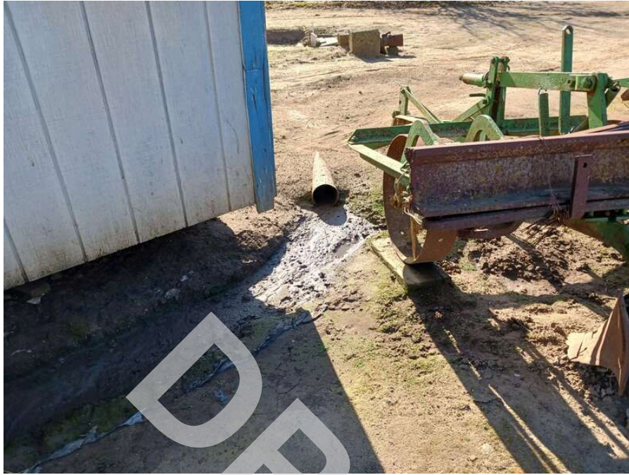
35. PVC piping connecting the sink to the "gray water" drainage system.
