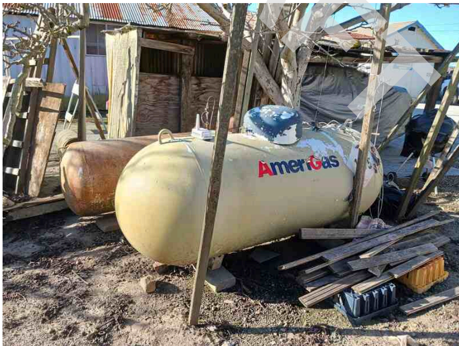
12. Propane tanks used to heat the main residential structure.
