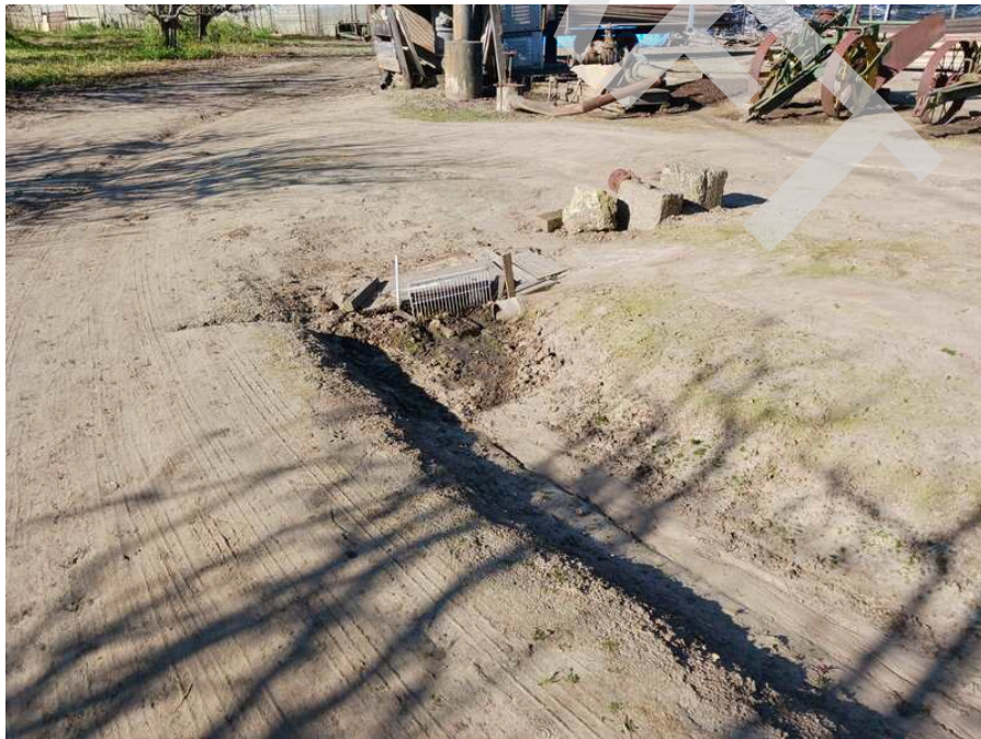
36. Termination point of "gray water" drainage system.
