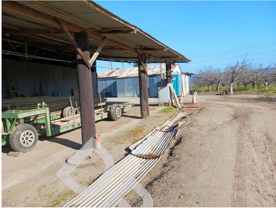
29. Overview of "gray water" drainage system.
