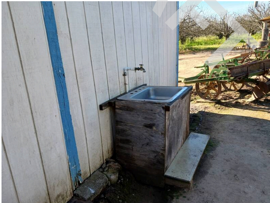
34. Sink attached to the "gray water" drainage system.
