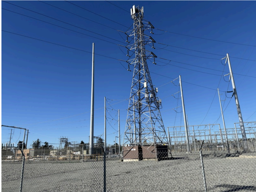
38. Adjacent PG&E Substation
