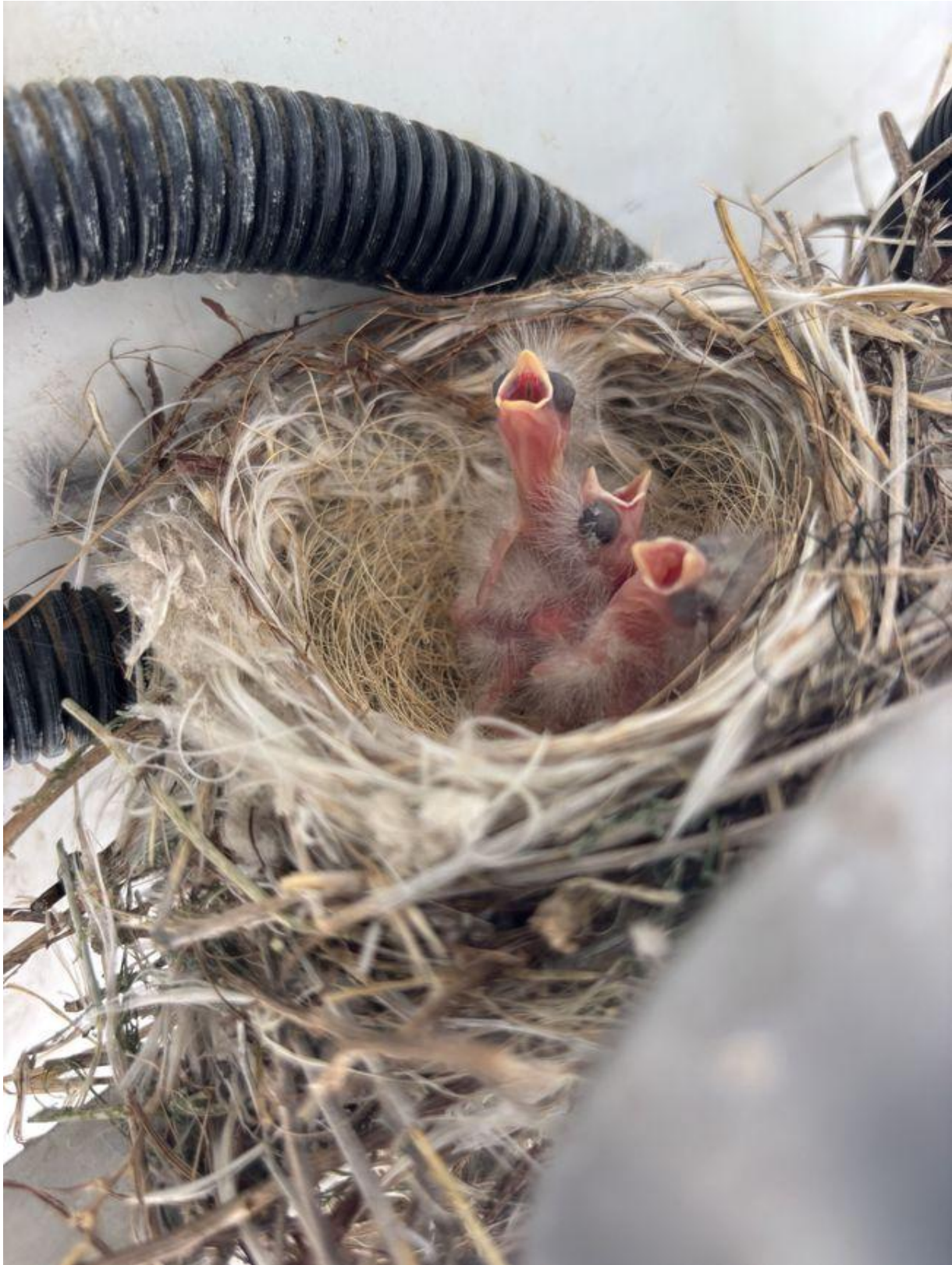
Nestlings inside nest above pressure valves.
