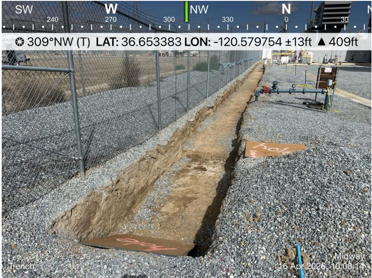
Trench with sufficient ramp and hole adequately covered, no gaps observed, for wildlife entrapment prevention.
