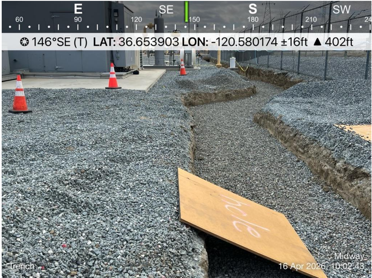
Trench with sufficient ramp and hole adequately covered, no gaps observed, for wildlife entrapment prevention.
