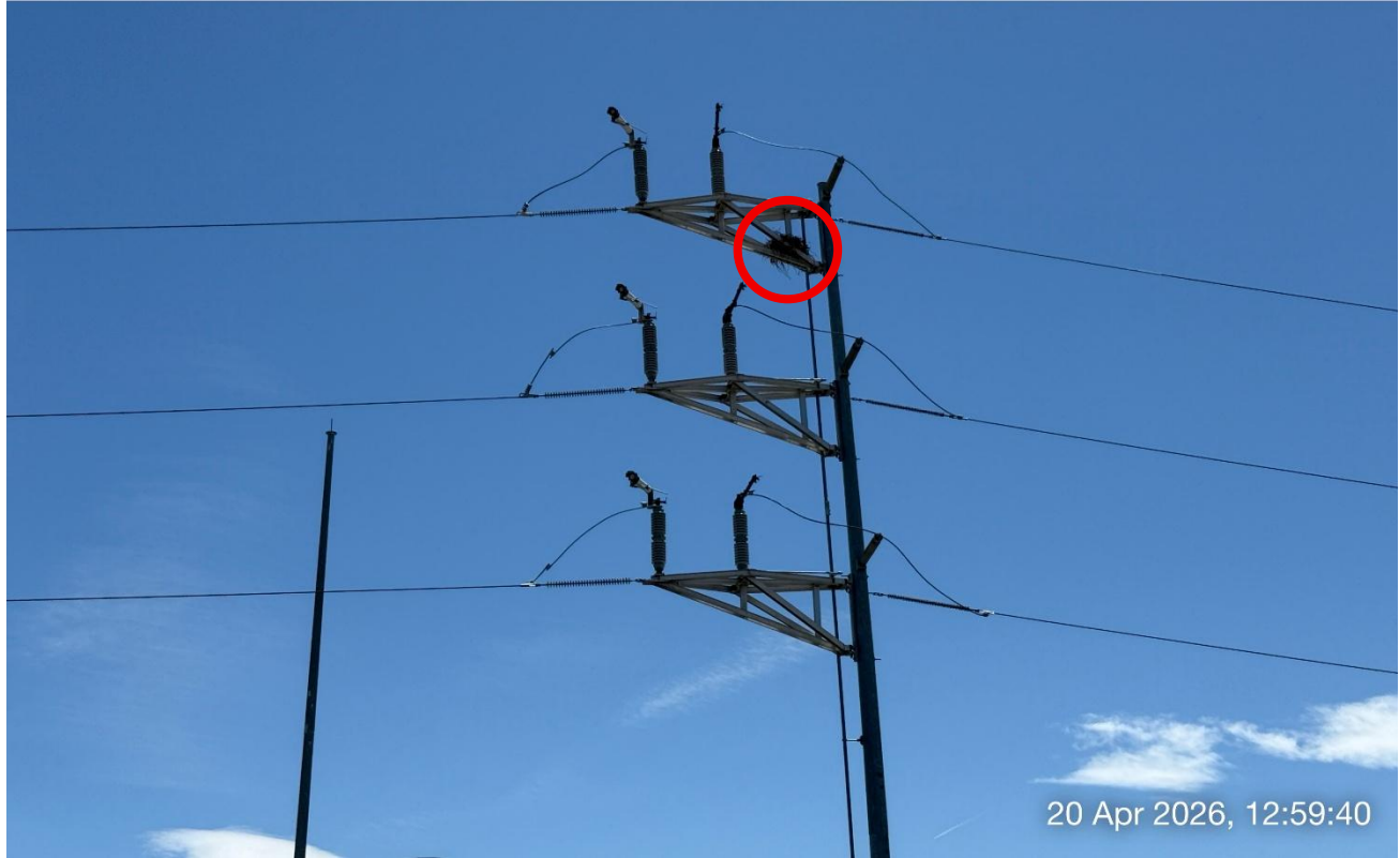
CORA nest in utility structure near gate at peaker plant
