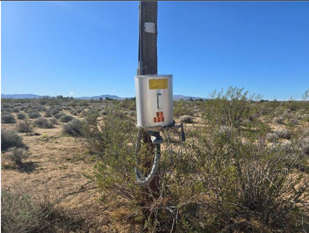
Photo 35: View of transformer on Subject Property along the southern boundary of the eastern portion of the Subject Property. BSK did not observe evidence of staining or stickers indicating PCB contents.
