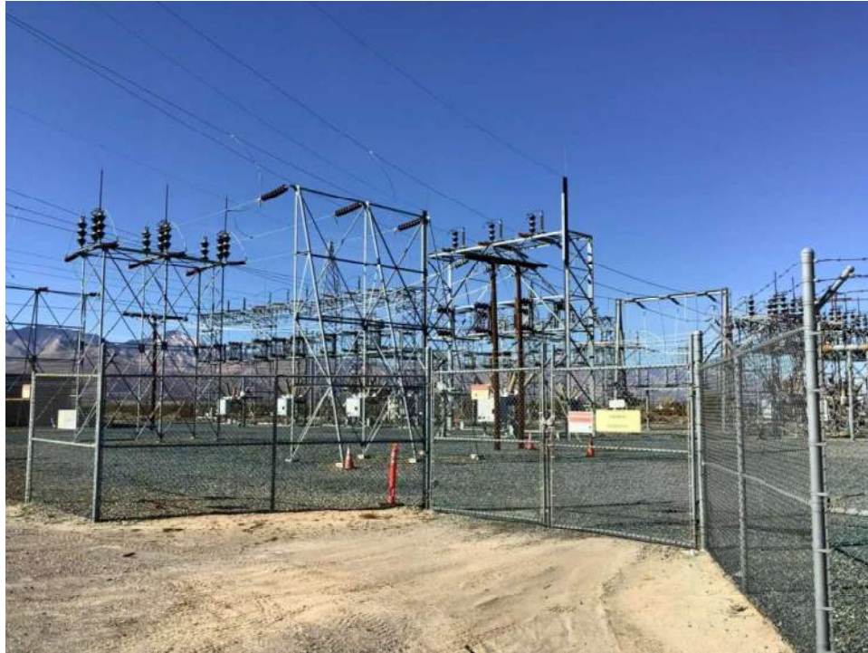
Photo 7. Detail of equipment, view toward northwest.
