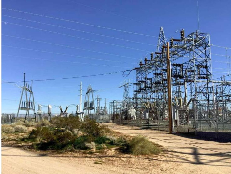
Photo 3. Western side of the substation, view toward northeast.
