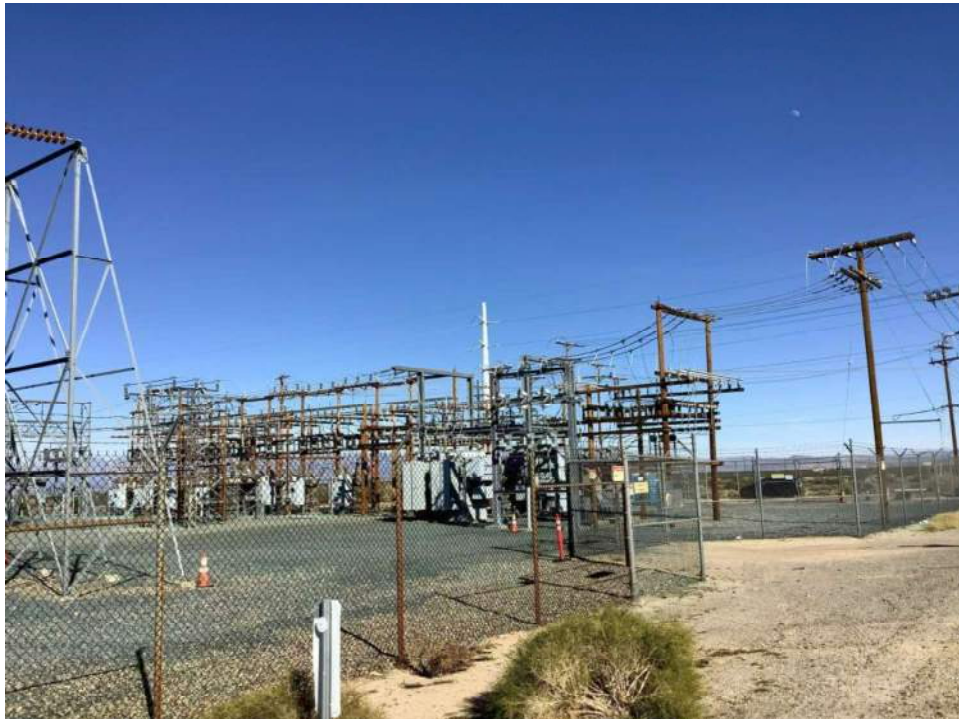
Photo 8. Detail of equipment, view toward northeast.
