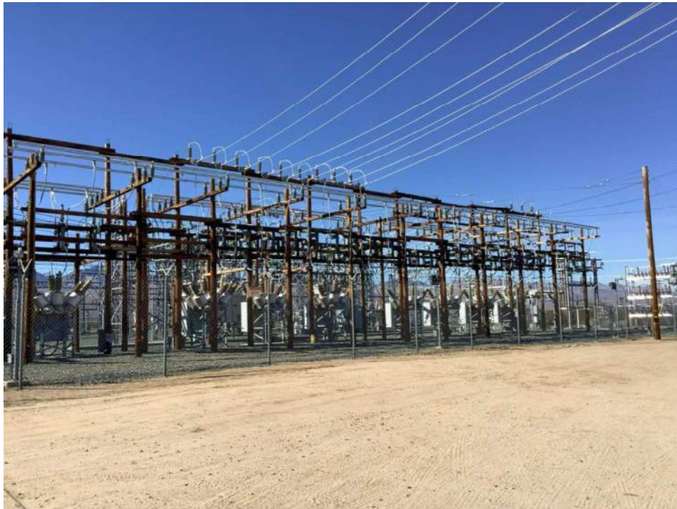
Photo 6. Detail of equipment, view toward northwest.
