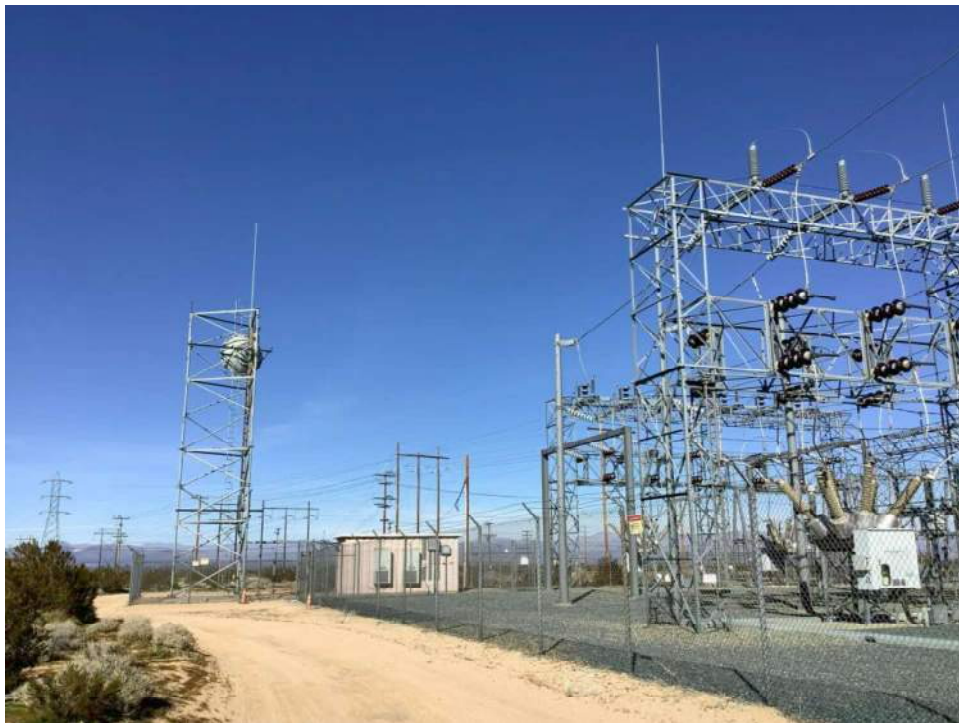
Photo 4. View of side area of substation, including the c.1960 shed. View toward northeast.
