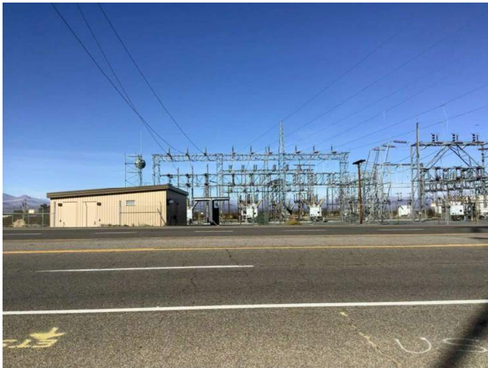
Photo 2. View of Inyokern substation from across Brown Road, with view of shed constructed c.2021. View toward north.
