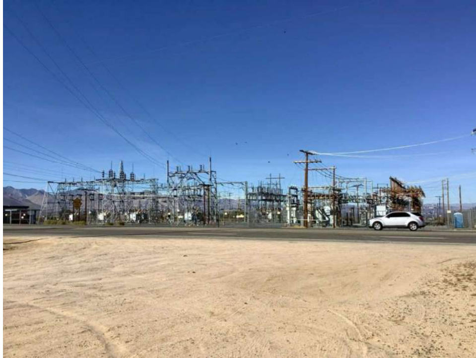
Photo 1. View of Inyokern substation from across Brown Road. View toward northwest.
