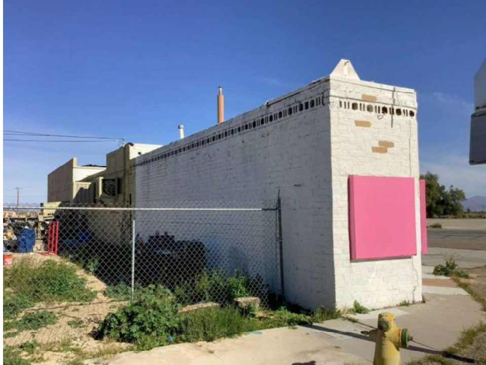
Photo 1. Side and rear façades, view toward northeast. This view reveals the odd shape of the building in response to the shape of the parcel.
