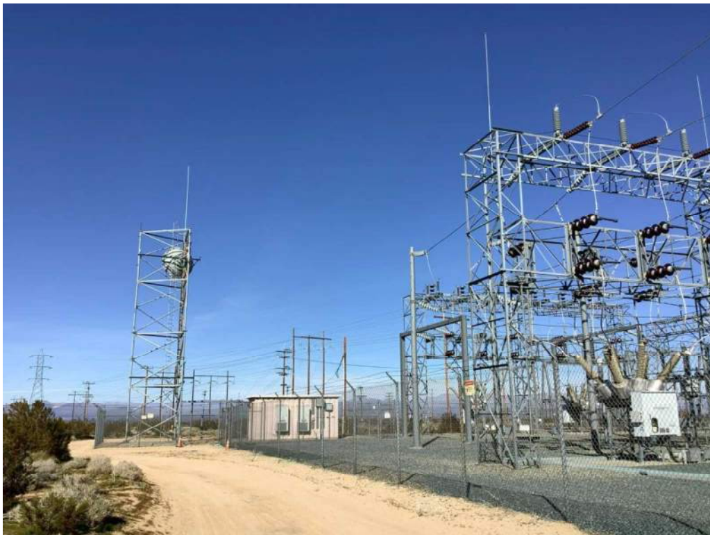
Figure 4.29.3 Inyokern Substation with mid-century shed in the center, view toward northeast.
