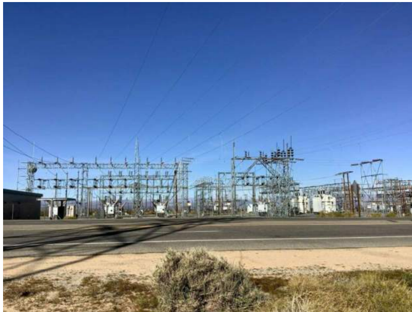
Figure 4.29.1 Inyokern Substation view north from Highway 178.
