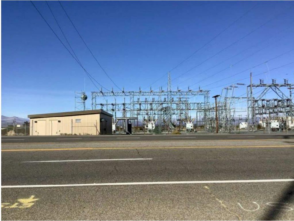
Figure 4.29.2 Inyokern Substation, with recent shed visible on the left. View toward north.
