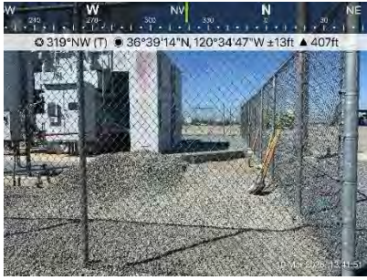
Gravel inside the transformer gate that was moved.
