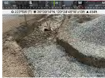
End of day, extent of hydrovacuuming for the day. Crew loaded gravel into dried section of the trench.
