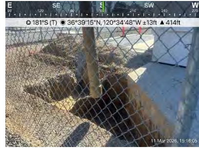
Box that was made, 3ft depth. Transformer is the box in the top right of the photo.
