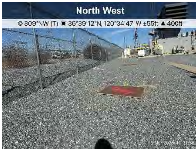
Potholes after they were excavated and covered for safety.
