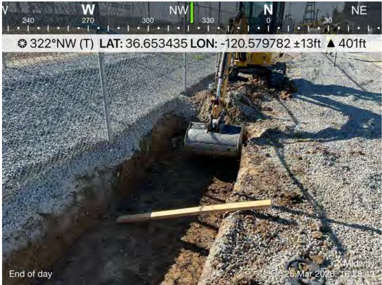
End of day sweep. Adequate ramp in trench for wildlife entrapment prevention.
