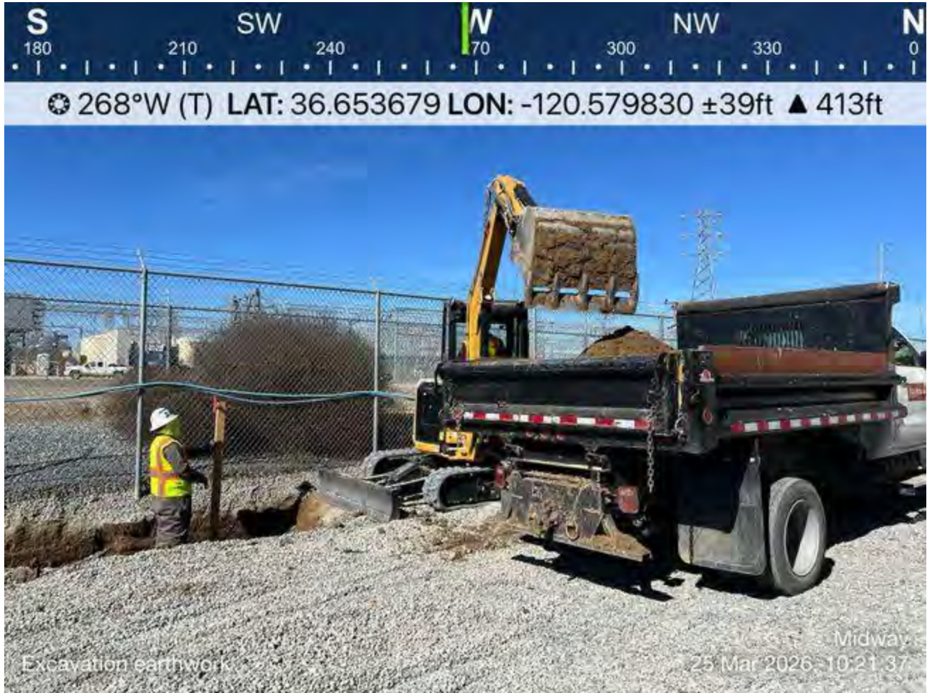
Trenching earthwork activities using a mini excavator, excavating directly onto truck for hauling.
