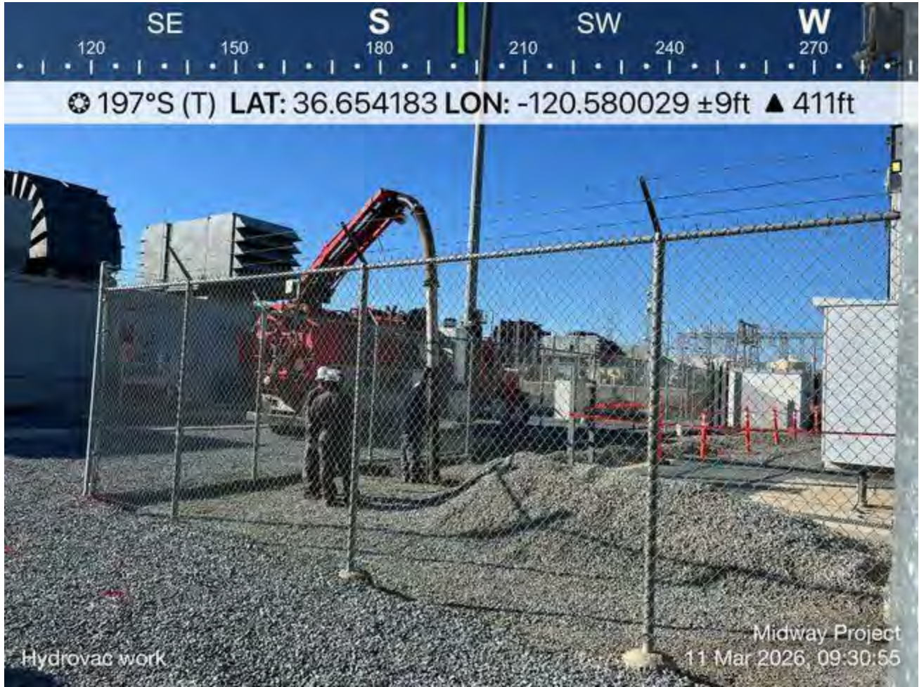
Hydrovac work activities, including hydrovac truck and handheld tools to shovel gravel to the side.
