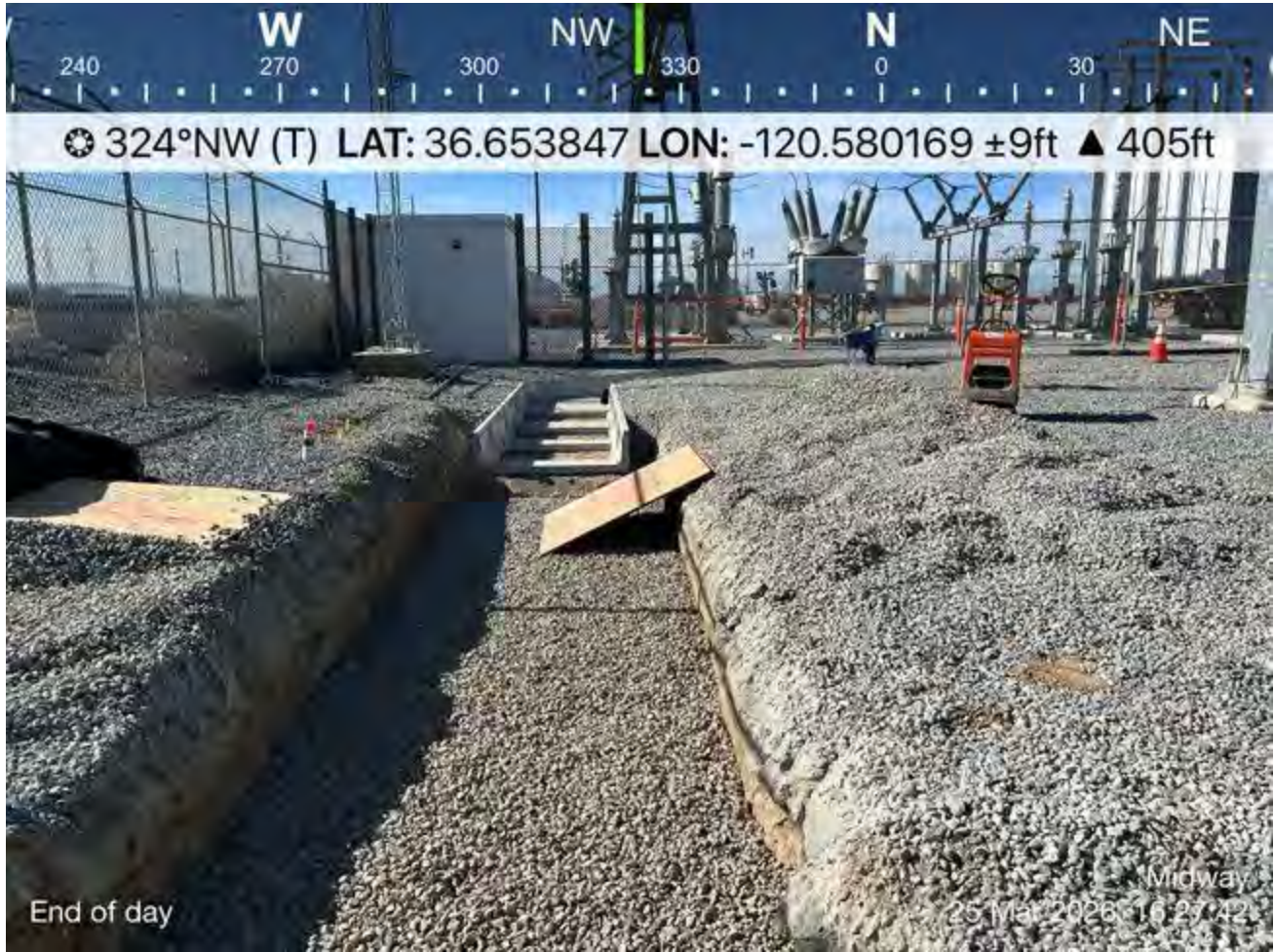
End of day sweep. Adequate ramp in trench and hole covered for wildlife entrapment prevention.
