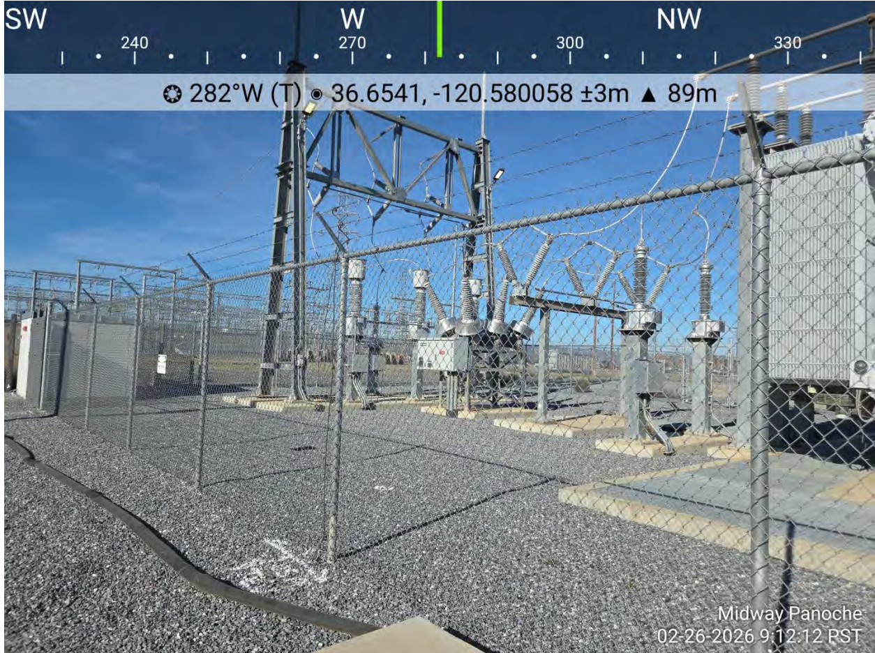
Gen-tie tie-in location
