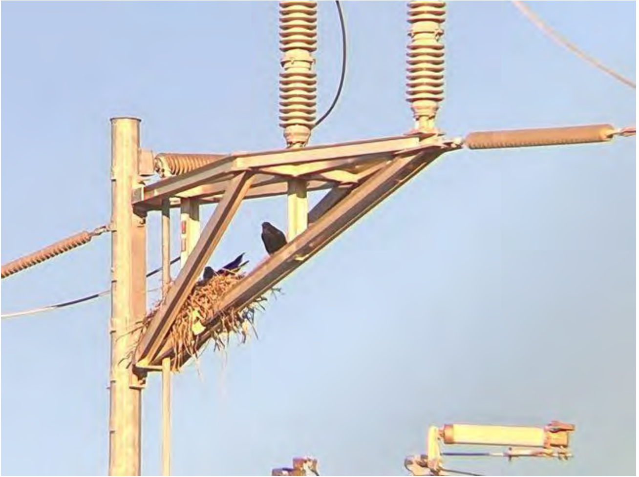
Common raven stick nest observed in electrical pole.
