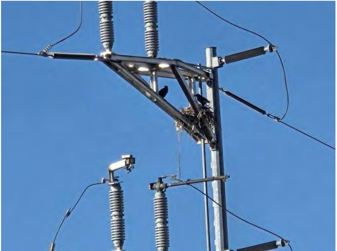
American crow nest in utility pole.
