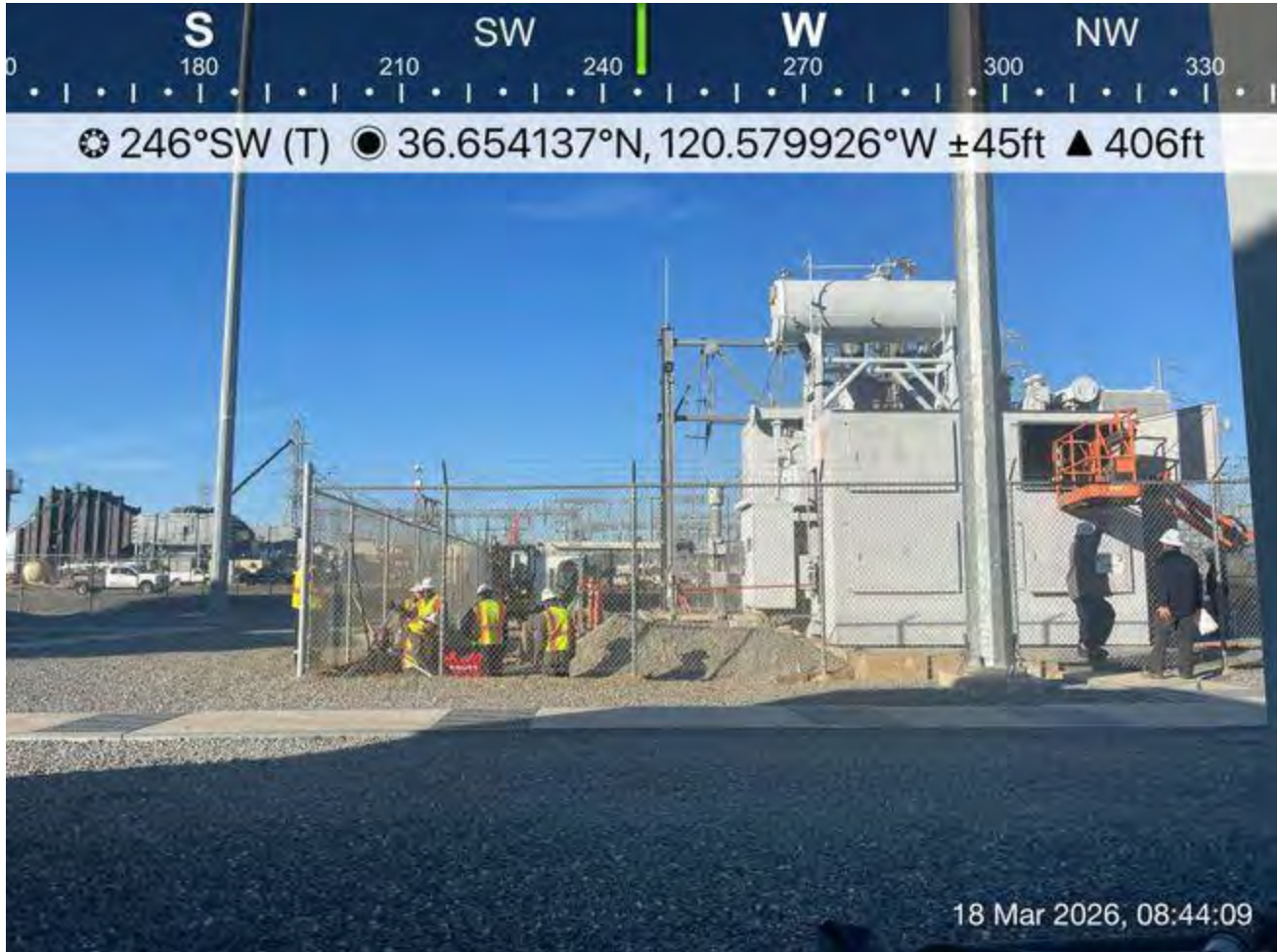
Section of fence removed and small excavator brought within the fence line.
