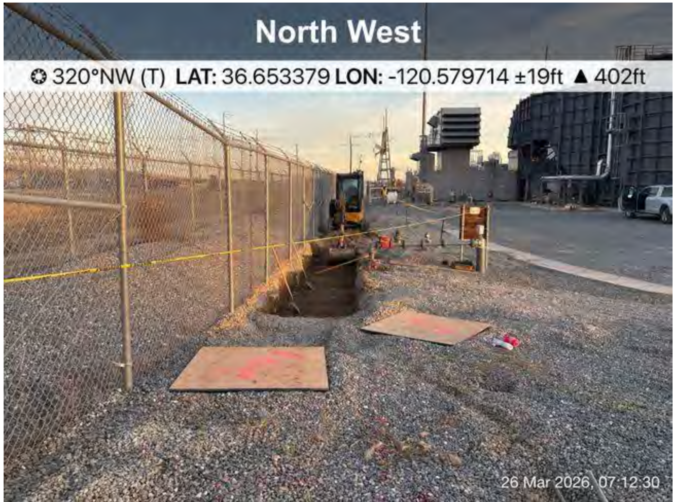
Work area during bio sweep of site. All ramps in trench were appropriate for wildlife to escape, if necessary.
