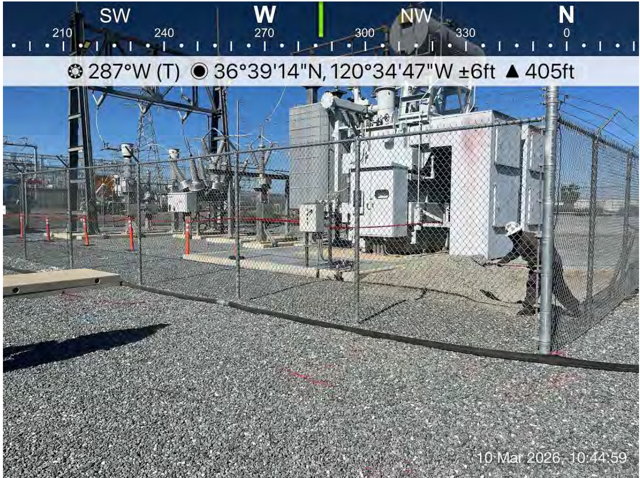
Photo 2: View of substation with installed safety buffer (red tape) and crews working to remove rock base.
