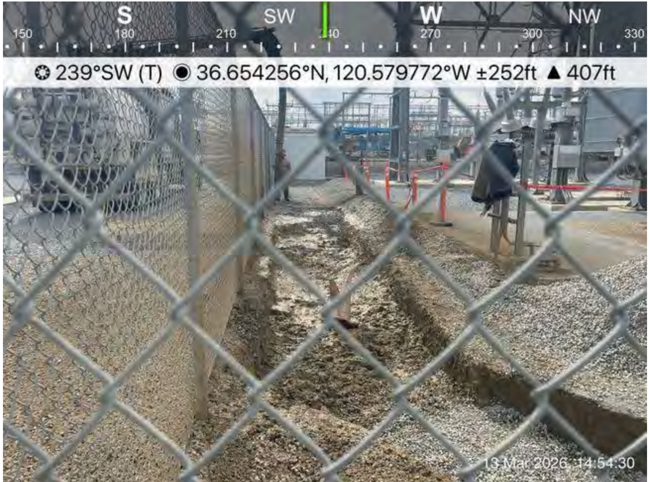
End of day check of open trench with earthen wildlife escape ramp
