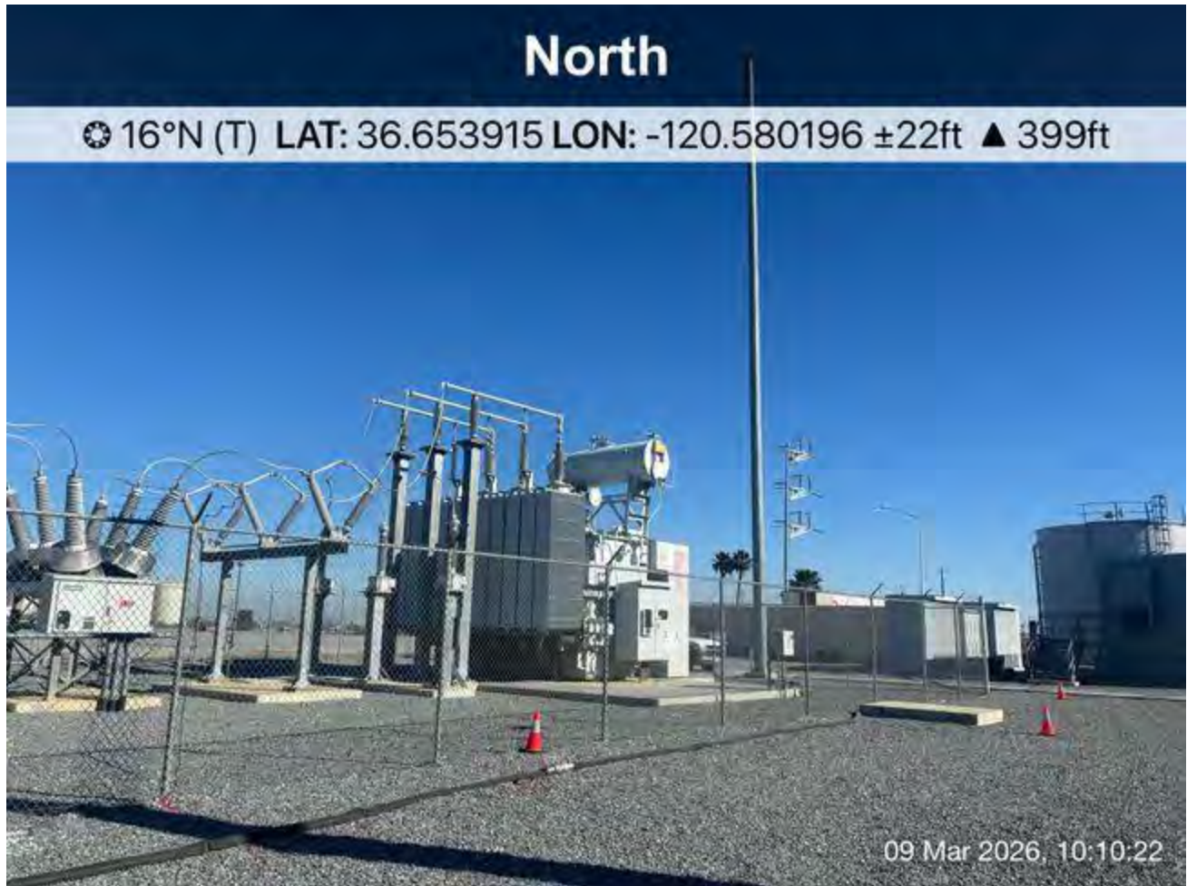
View of transformer (nesting area) with nest buffer (cones) in place.
