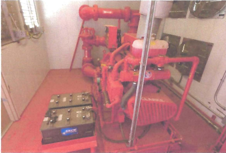
S-6 Emergency Fire Pump
