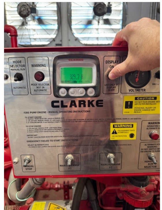
S-6 Fire Pump Engine Hours
