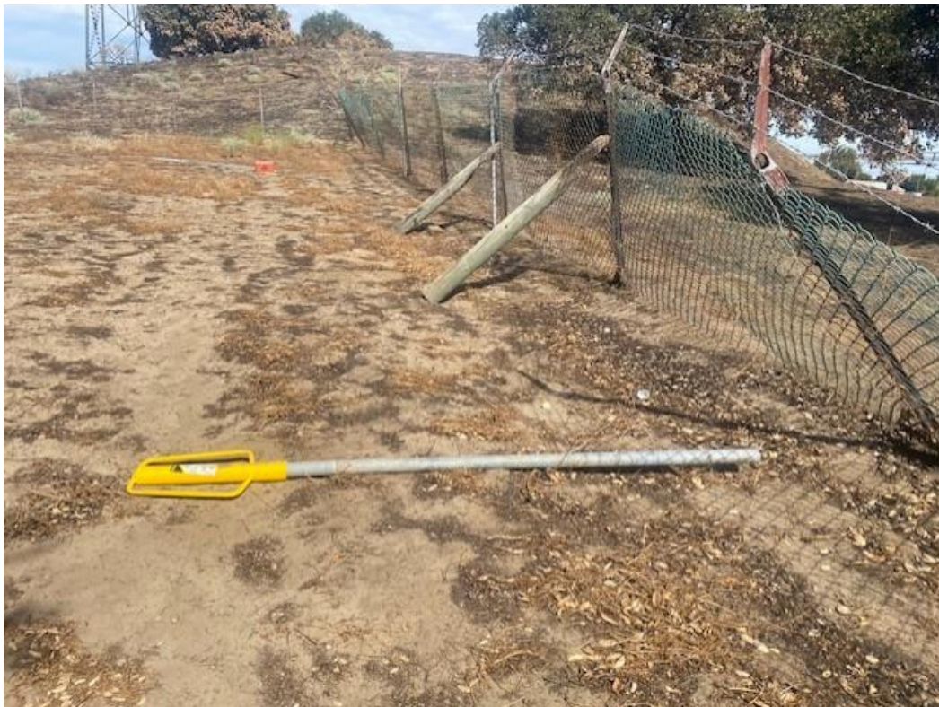
Photo 4. Chain link fence falling down along the East side of the Sardis Unit.
