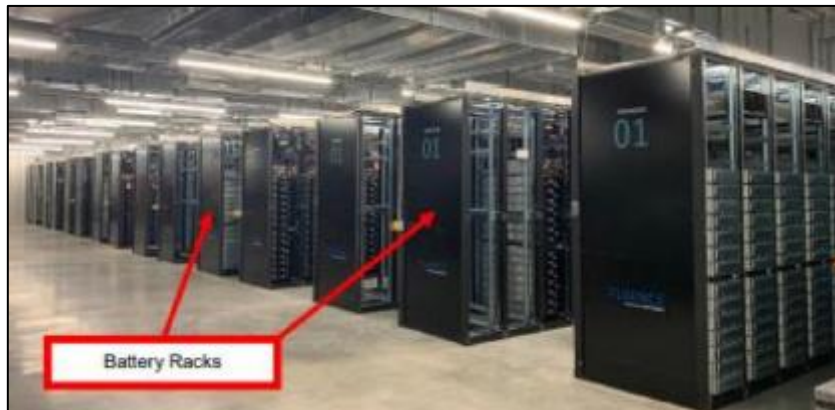
Figure 19 Interior battery rack setup of Chandler, Arizona facility
