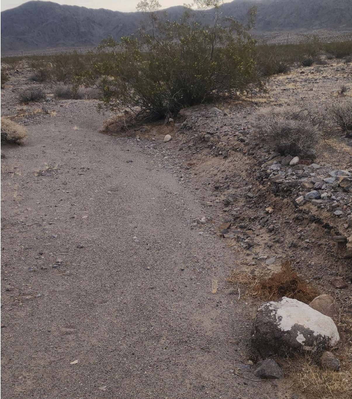
Photo Point T12 (Gen-Tie Corridor). East facing representative photograph illustrating indicators of an OHWM in a drainage feature, corresponding to ATG-005 Datasheet.
