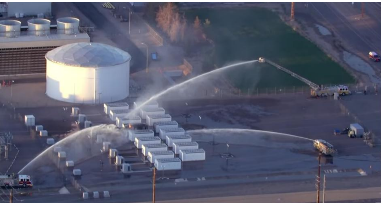
Figure 2. Firefighters Responding to the Peoria BESS Fire on October 1, 2025.
