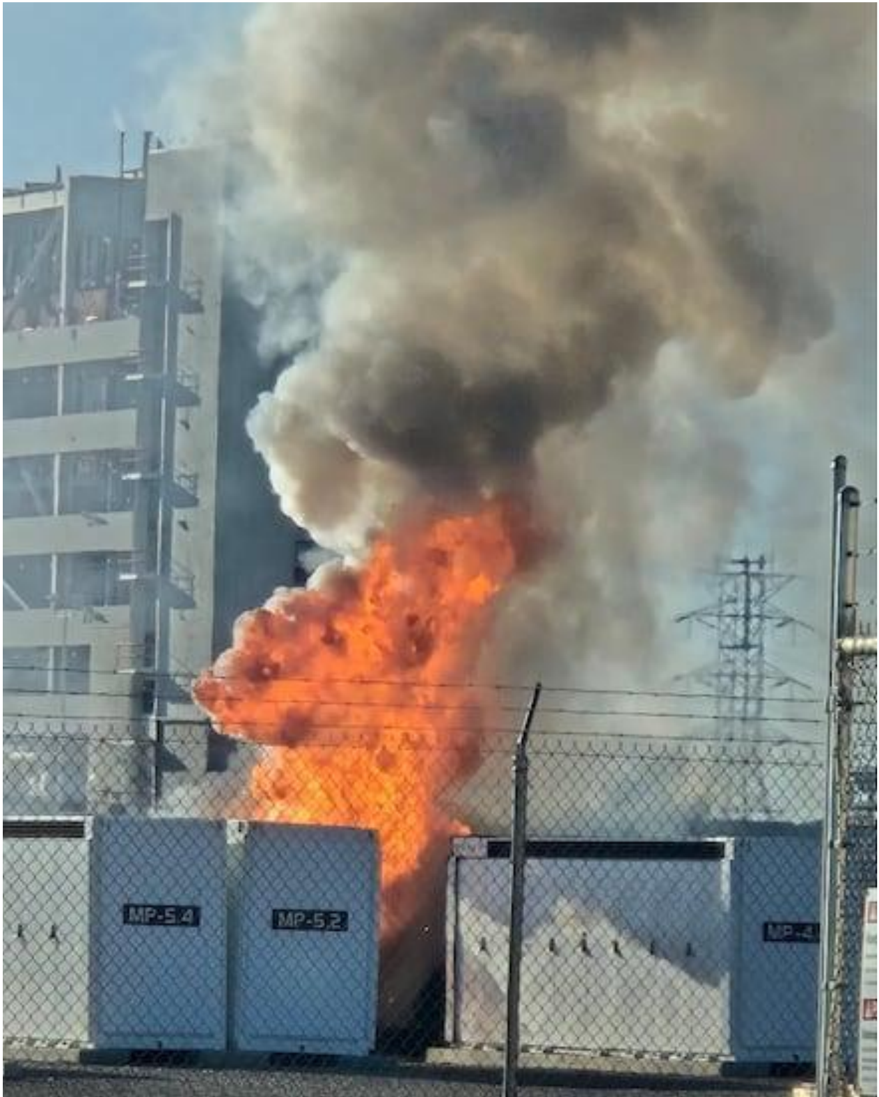
Figure 1. BESS Fire on October 1, 2025 in Glendale, Arizona.
