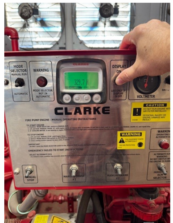
S-6 Fire Pump Engine Hours
