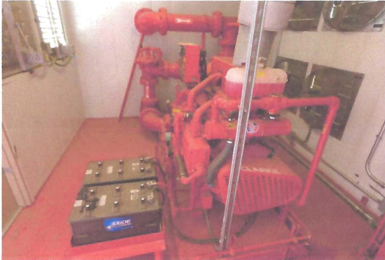
S-6 Emergency Fire Pump
