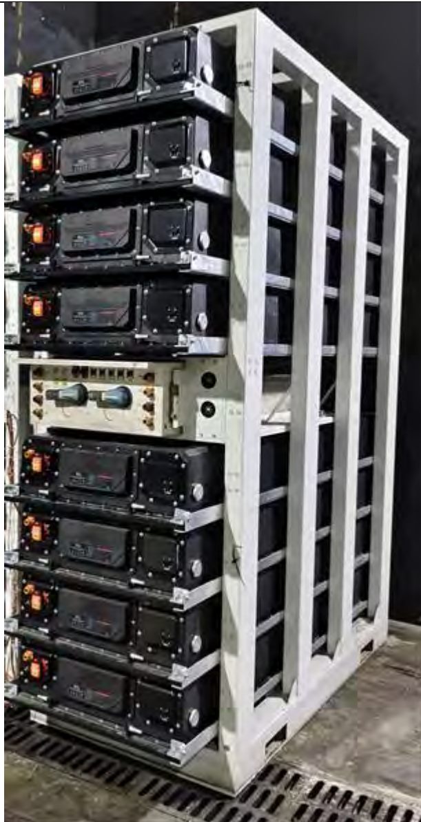
Figure 5. View 01 of battery systems
