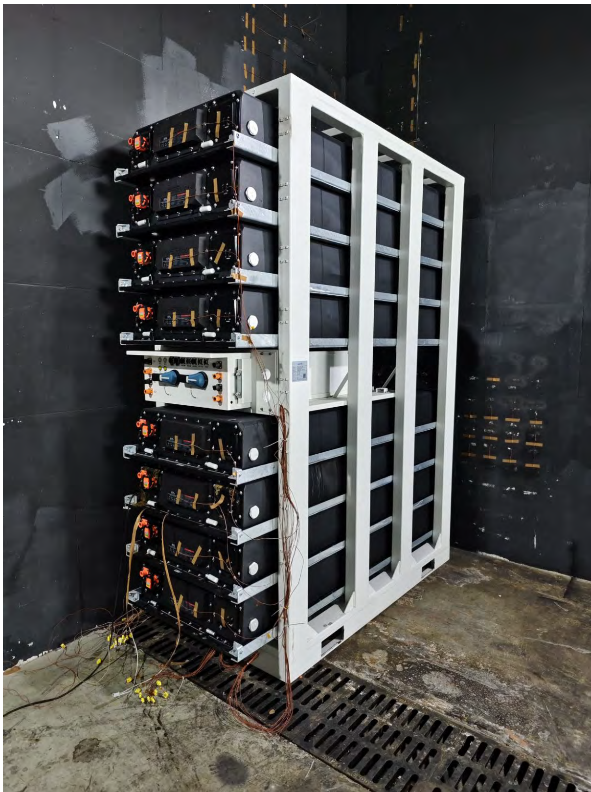
Figure 26. Photo 1 of initiating BESS Unit after test
