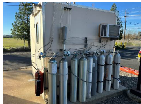
Photograph Number: 14 Date of Photograph: January 7, 2025 Direction of Photograph: South Description of Photograph: View of the Continuous Emissions Monitoring System (CEMS) shack and associated gas cylinders in the southern portion of the power plant.
