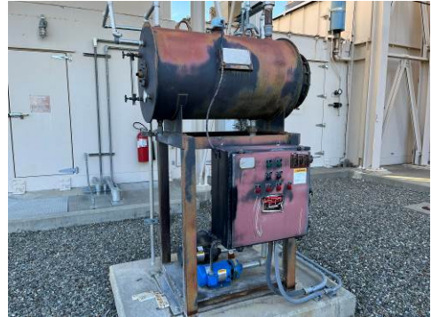
Photograph Number: 13 Date of Photograph: January 7, 2025 Direction of Photograph: East Description of Photograph: View of 30-gallon evaporative cooling water overflow AST located in the western portion of the power plant.
