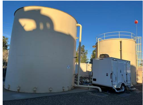
Photograph Number: 7 Date of Photograph: January 7, 2025 Direction of Photograph: Northwest Description of Photograph: View of two 44,000-gallon water ASTs (left: fire suppression, right: process water) process water ASTs located in the northwest portion of the power plant.
