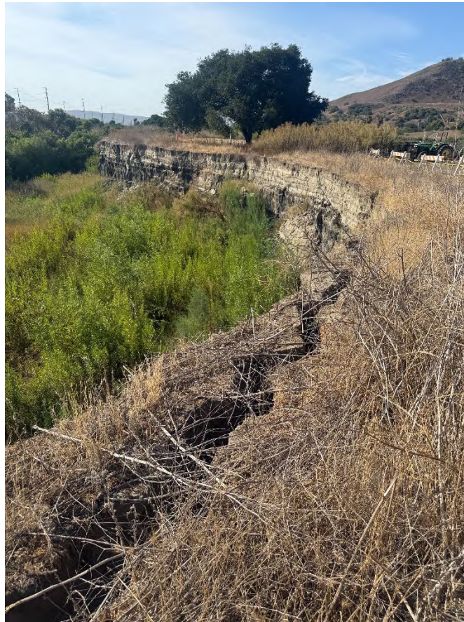
Figure 8 | Surface Cracks Along Channel Banks
